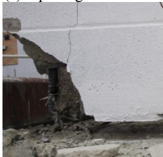
(c) Fracture at north end
