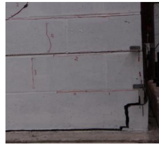
(b) Spalling at south end
