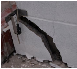
(a) Spalling at north end
