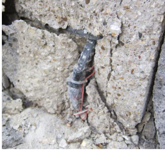
Figure 6-18 Buckling of longitudinal bars at south end of Specimen PBS-11 ( 8\Delta y )
