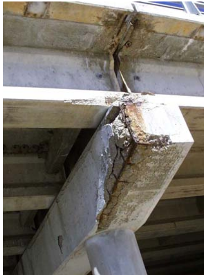
Figure 1.2 Concrete Spalling from Bridge Bent in Lubbock, Texas
