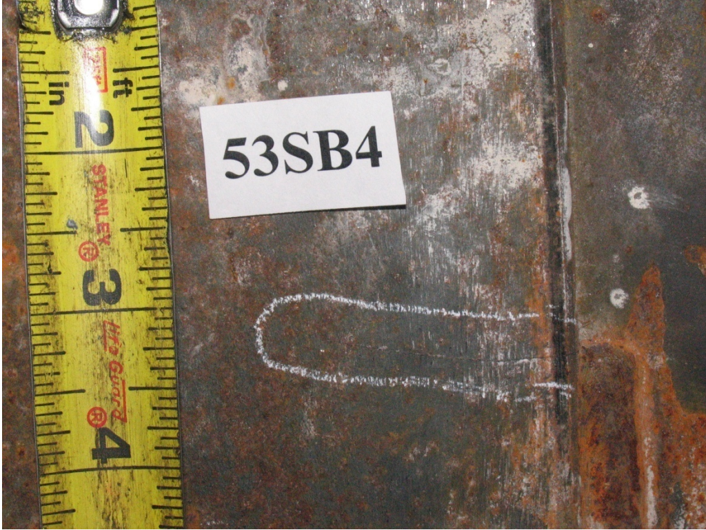
Figure 48. 53SB Failure Close-Up
