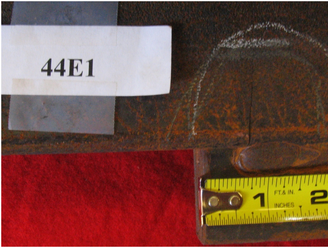
Figure 39. 44E Angle Failure Close-Up
