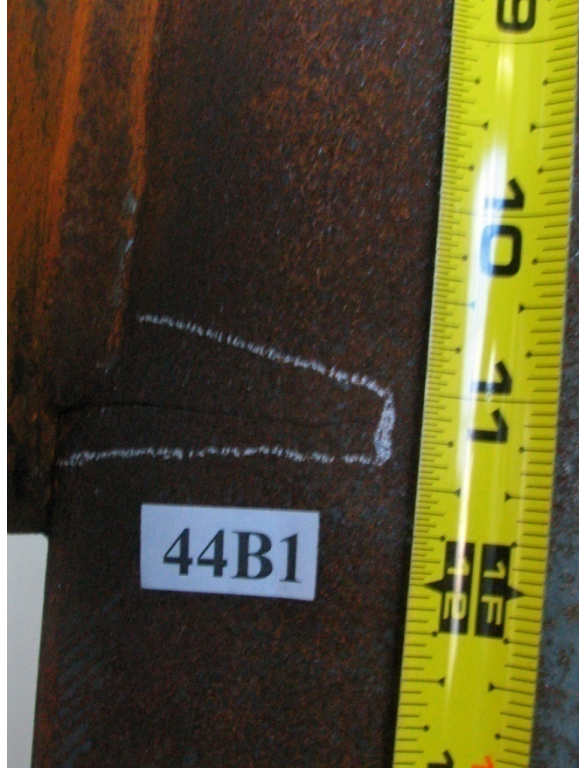
Figure 42. 44B Angle Failure Backside Close-Up
