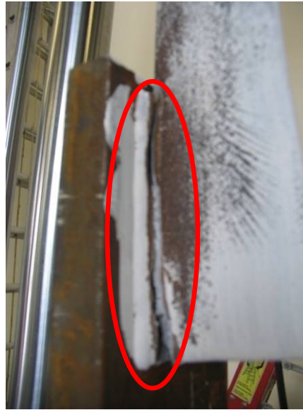
Figure 32. Typical Static Failure of Weld
