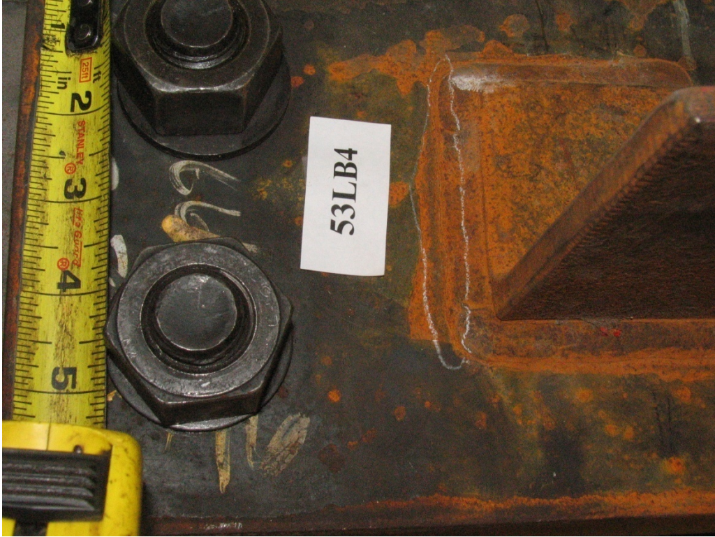
Figure 53. 53LB Angle Failure Close-Up
