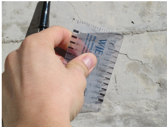
Figure A-80 – Shear crack (0.01 inches) (a in Figure A-79)
