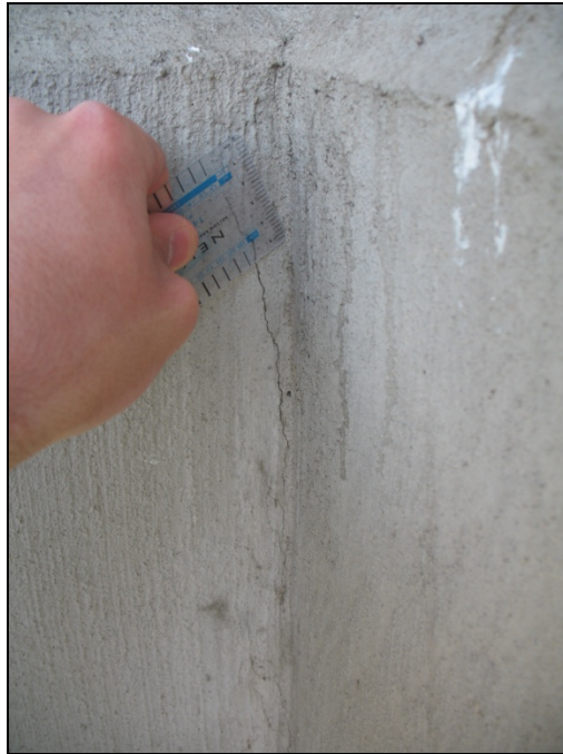
Figure A-22 - Cracking along ledge-step interface (a in Figure A-21)
