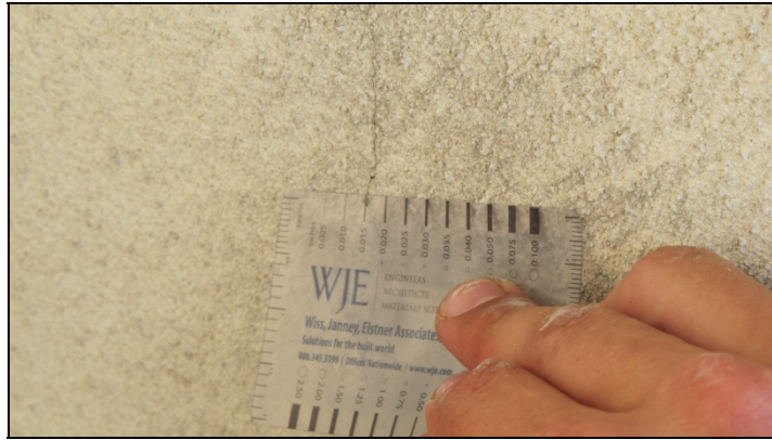
Figure A-37 - Shear crack (0.015 inches) (b in Figure A-35)
