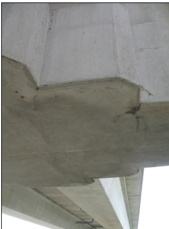
Figure A-12 - Crack on base of cap (b in Figure A-10)
