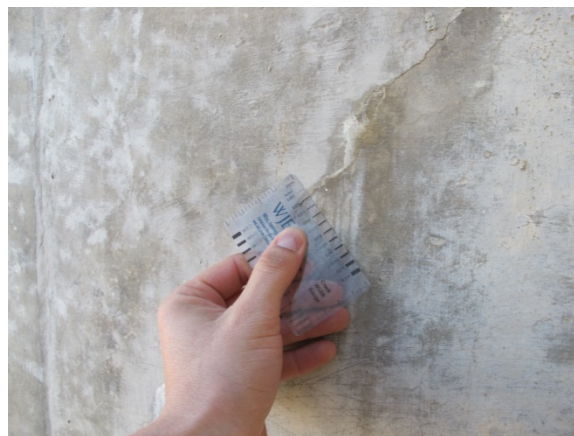
Figure A-84 - Shear crack (0.01 inches) (a in Figure A-83)
