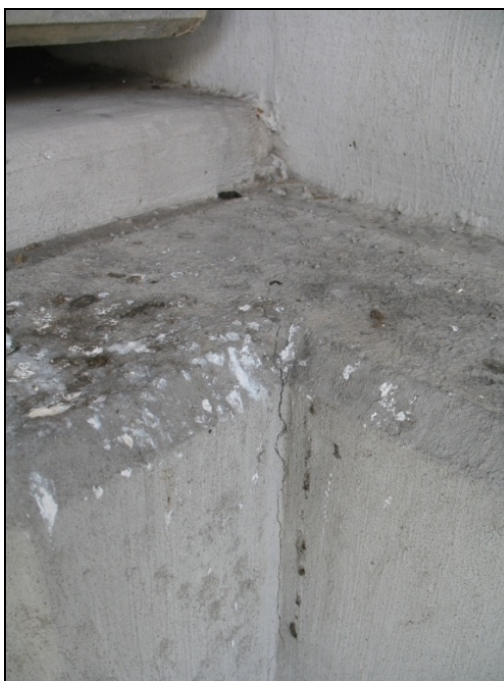
Figure A-11 - Ledge cracking (a in Figure A-10)
