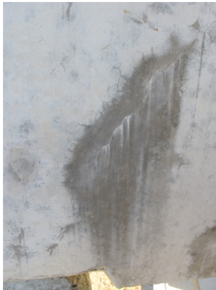
Figure A-65 - Shear crack (0.01 inches) extending from the edge of the column (a in Figure A-64)
