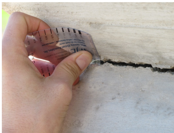
Figure A-70 – Cracking between the column and beam (0.375 inches) (a in Figure A-69)
