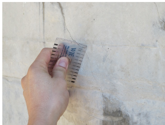
Figure A-60 – Shear crack (0.005 inches) (a in Figure A-59)
