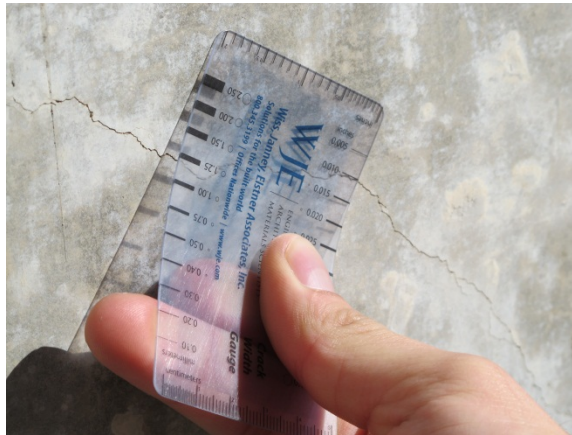
Figure A-81 – Shear crack (0.01 inches) (b in Figure A-79)
