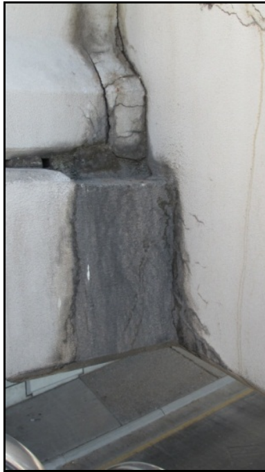
Figure A-41 – Water damage and cracking along web-ledge interface (b in Figure A-39)
