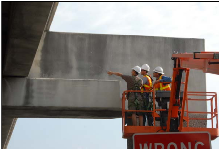
Figure A-1 - Bucket truck allowed for close observation of the crack
