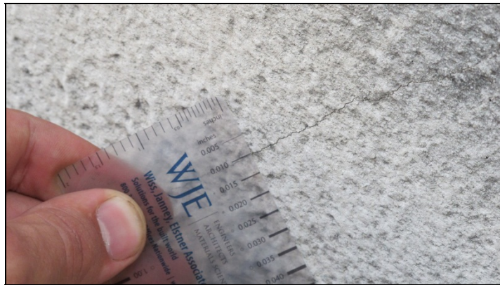
Figure A-34 - Moment crack (0.01 inches) (b in Figure A-32)
