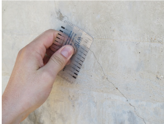
Figure A-61 - Shear crack (0.01 inches) (b in Figure A-59)
