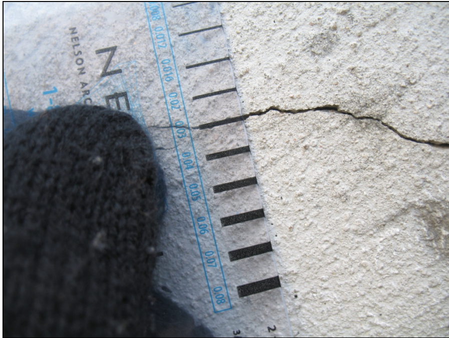
Figure A-18 – Largest shear crack (0.03 inches) (a in Figure A-17)
