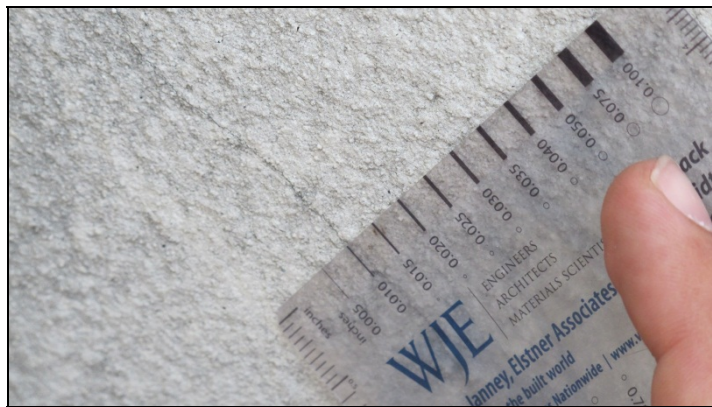
Figure A-29 - Shear crack (0.01 inches) (a in Figure A-28)
