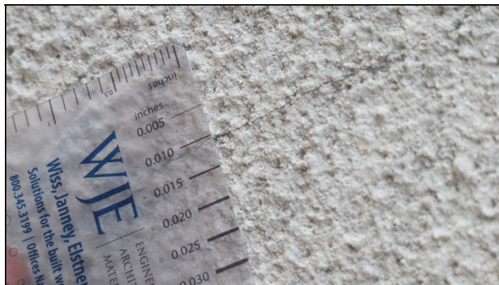
Figure A-30 - Moment crack (0.01 inches) (b in Figure A-28)
