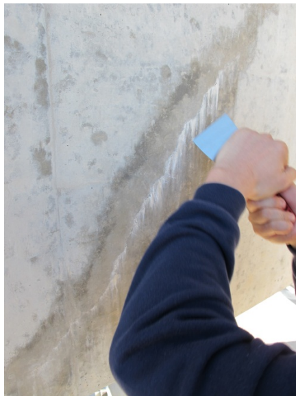
Figure A-56 – Efflorescence scraped off beam before crack widths were measured
