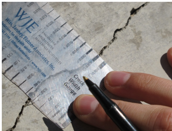
Figure A-82 – Cracking along column-beam interface (c in Figure A-79)
