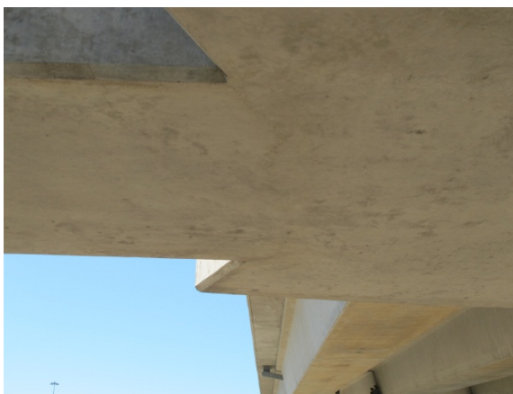
Figure A-73 - Crack extending through the entire width of the beam (d in Figure A-69)
