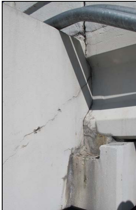
Figure A-49 - Water damage and cracking along web-ledge interface (d in Figure A-45)
