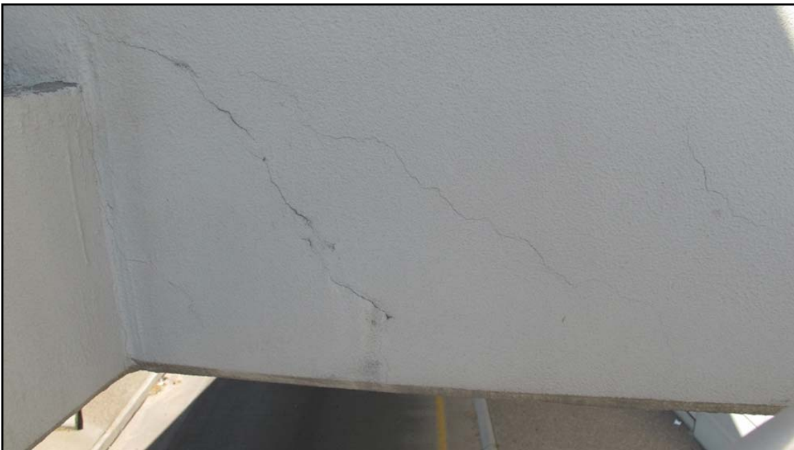
Figure A-54 - Shear crack and web-ledge interface crack (a in Figure A-53)
