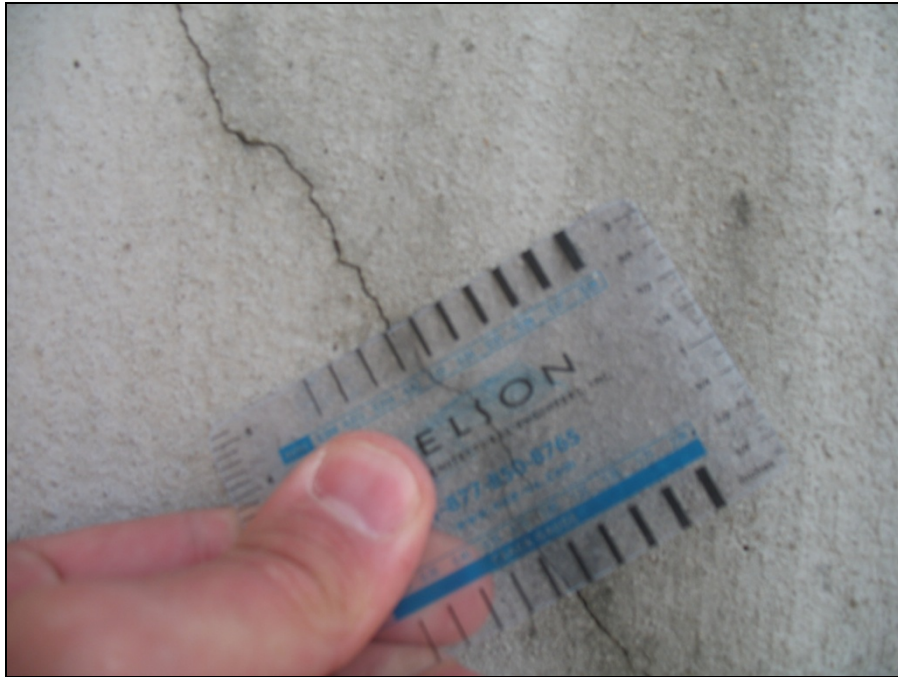
Figure A-24 – Largest shear crack (0.02 inches) (c in Figure A-21)
