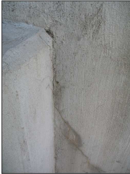
Figure A-25 - Cracking at web-ledge interface (d in Figure A-21)
