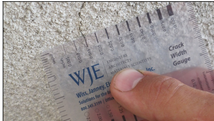
Figure A-36 - Shear crack (0.015 inches) (a in Figure A-35)
