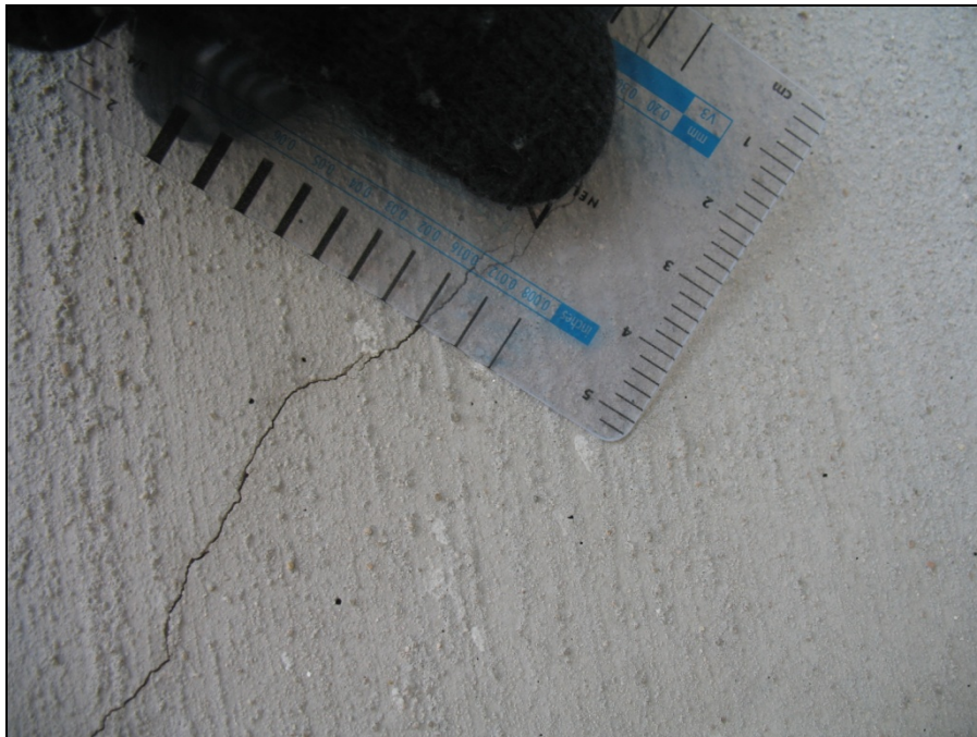
Figure A-19 – Crack above ledge (0.016 inches) (b in Figure A-17)
