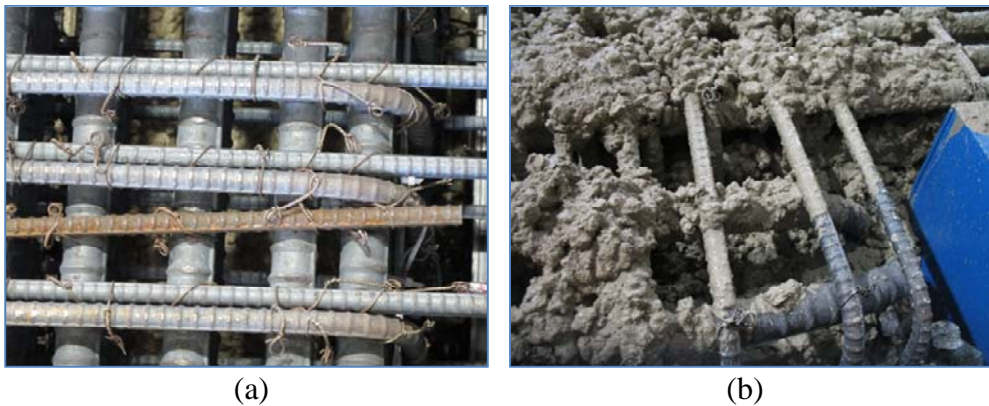
Figure 3-20: Congested reinforcement cages
