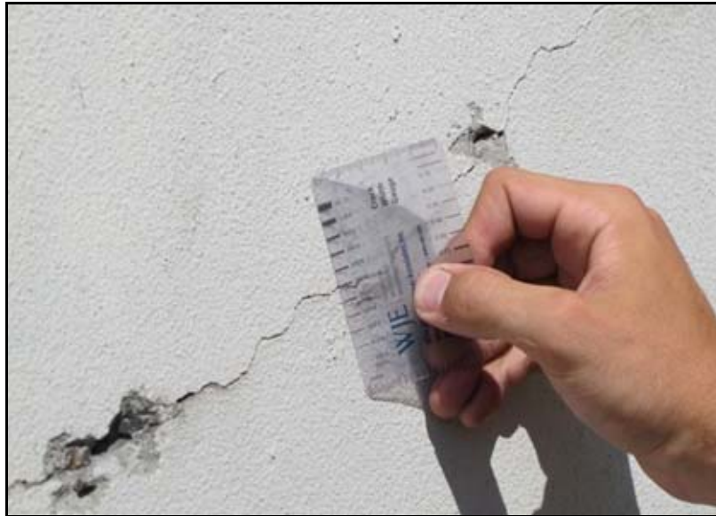
Figure A-48 - Shear crack (0.03 inches) and spalling (c in Figure A-46)
