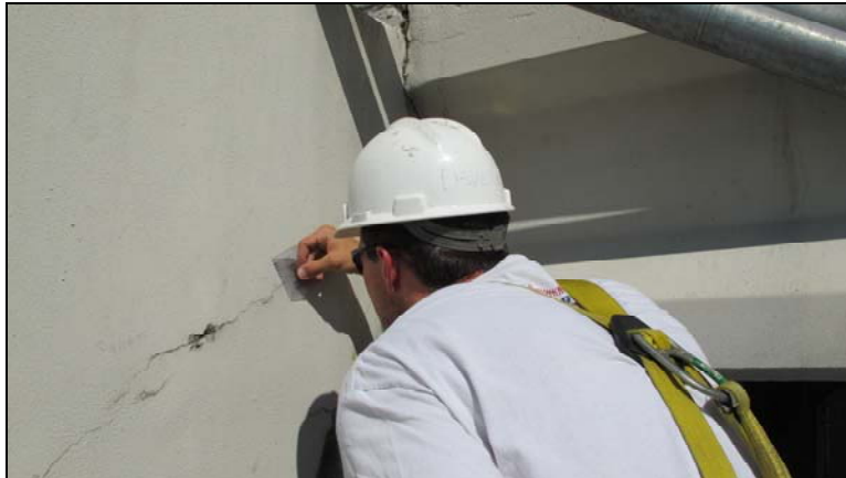
Figure A-2: Cracks were measured using crack gauge and recorded
