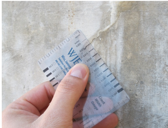
Figure A-85 - Shear crack (0.01 inches) (b in Figure A-83)
