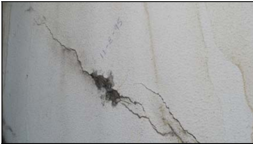
Figure A-40 - Largest shear crack (0.04 inches) and spalling (a in Figure A-39)
