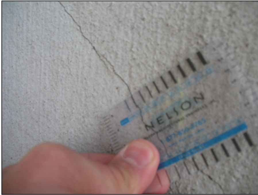
Figure A-26 – Crack above ledge (e in Figure A-21)
