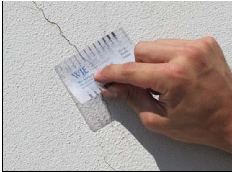
Figure A-46 - Moment crack (0.02 inches) (a in Figure A-45)
