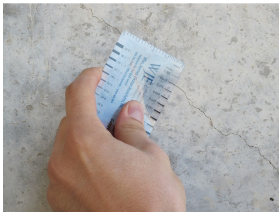
Figure A-75 – Shear crack (0.01 inches) (a in Figure A-74)
