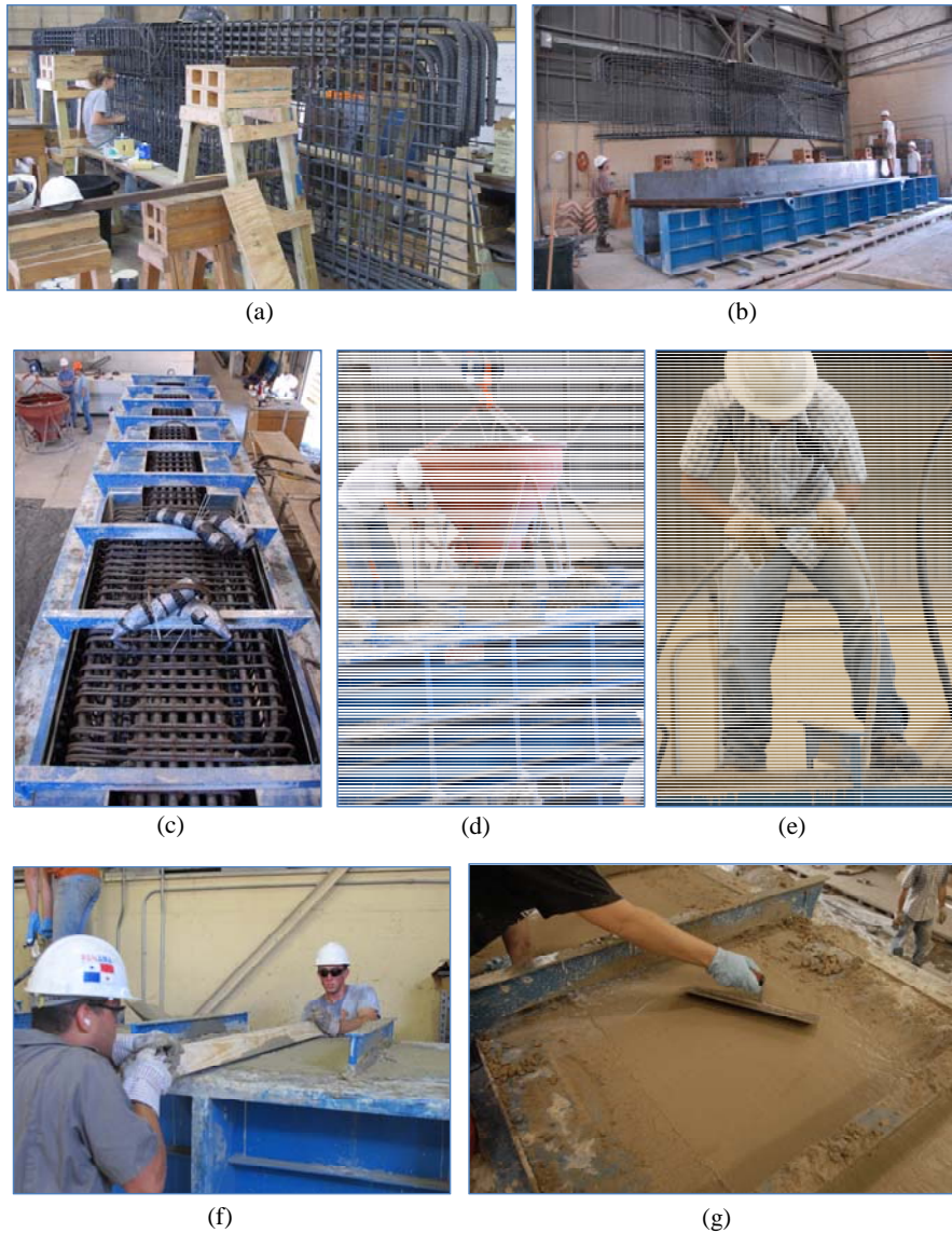
Figure 3-19: Fabrication of a typical specimen; (a) Construction and instrumentation of cage, (b) fully instrumented reinforcement cage being dropped in formwork, (c) reinforcement cage in the fully assembled formwork, (d) concrete bucket used in concrete placement, (e) internal vibration used to ensure proper consolidation, (f) screeding to obtain a proper concrete level, (g) troughs were used to finish the top of the specimen
