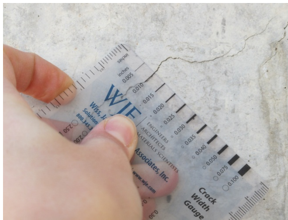
Figure A-86 - Shear crack (0.01 inches) (c in Figure A-83)
