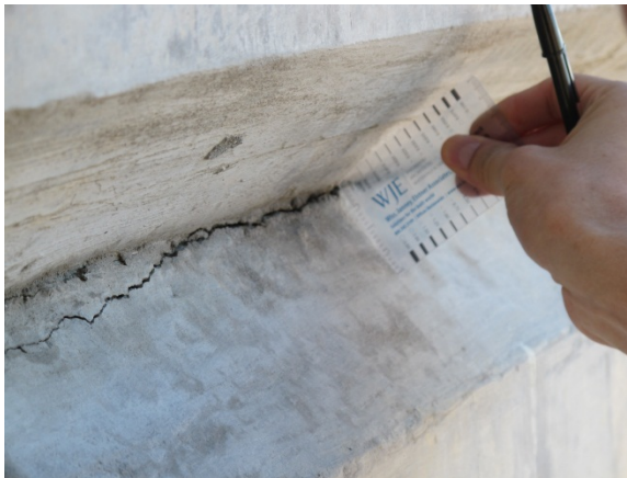
Figure A-77 – Cracking along column-beam interface (c in Figure A-74)
