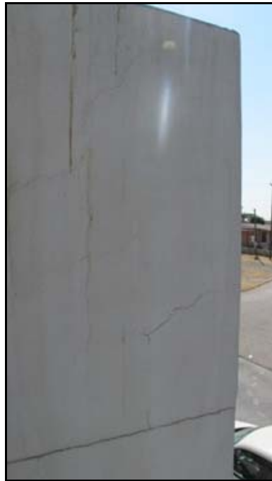
Figure A-44 - Moment cracking (e in Figure A-39)
