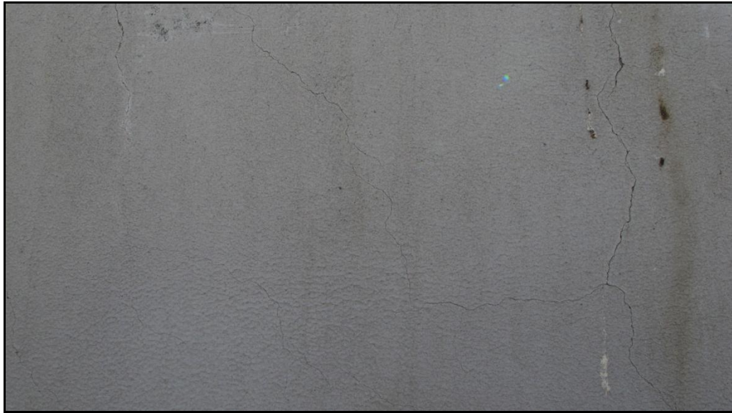
Figure A-43 - Map cracking located in the middle of shear span (d in Figure A-39)
