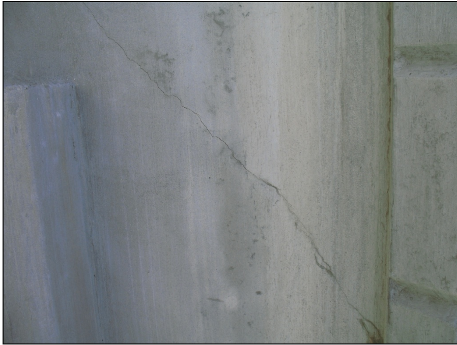
Figure A-6 – Largest shear crack (0.02 inches) (a in Figure A-5)
