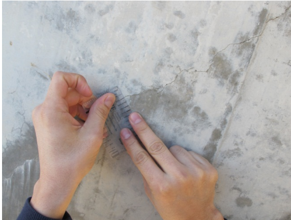
Figure A-66 – Shear crack (0.01 inches) (b in Figure A-64)
