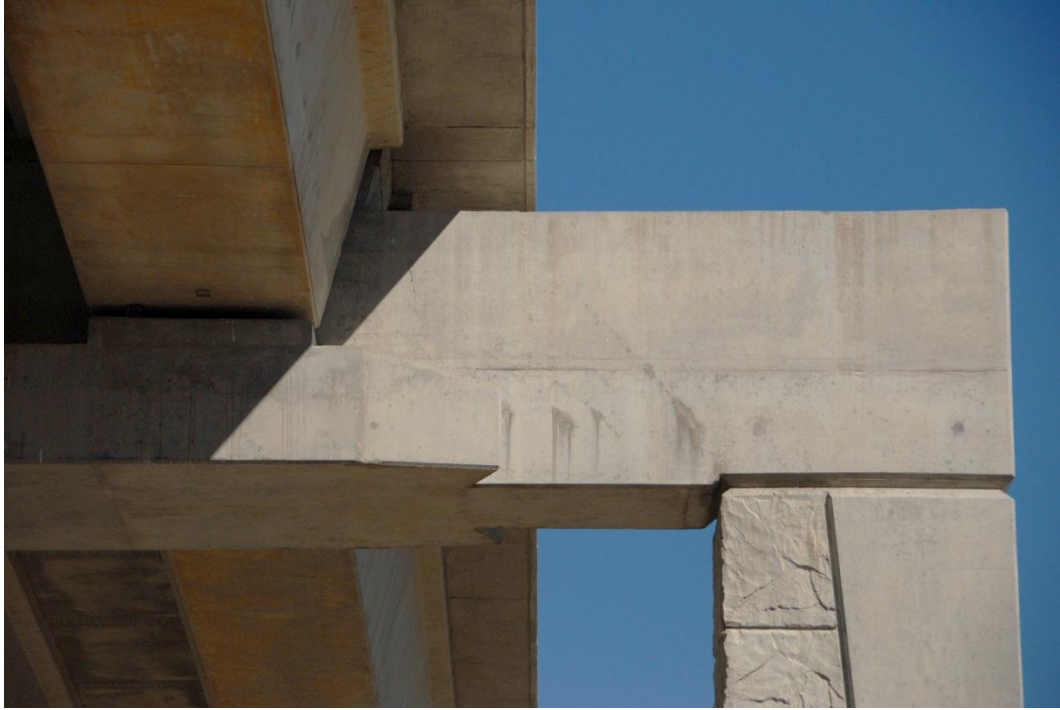
Figure A-63 – Overall view of SE corner of Bent 17
