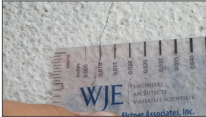
Figure A-33 -Shear crack (0.01 inches) (a in Figure A-32)
