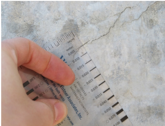
Figure A-71 – Shear crack (0.005 inches) (b in Figure A-69)
