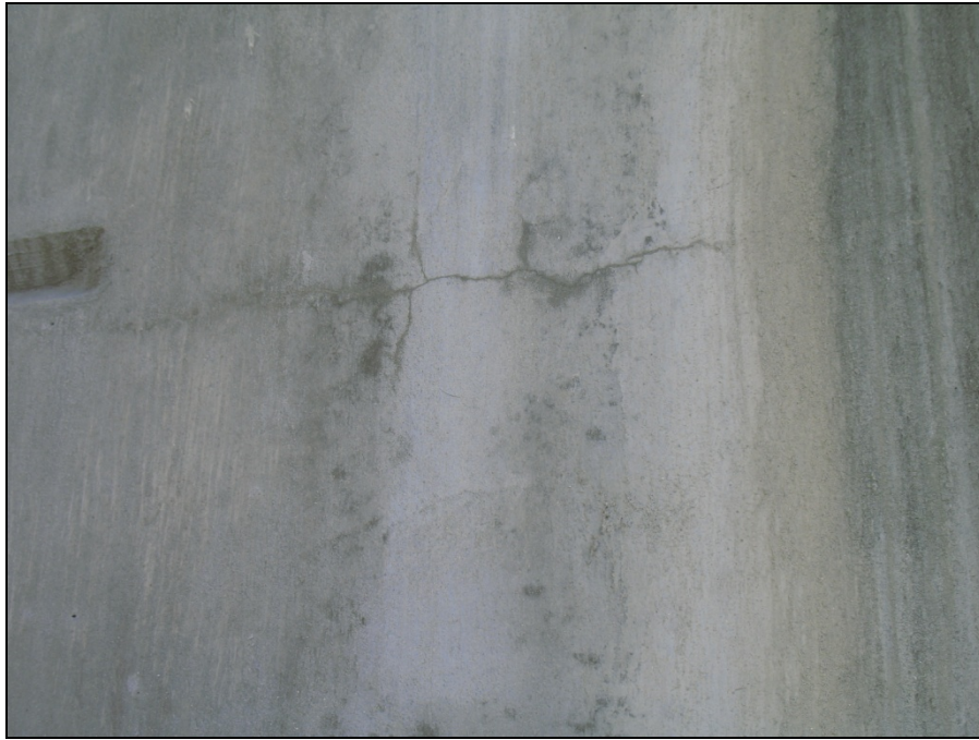
Figure A-8 – Horizontal cracking above shear crack (c in Figure A-5)
