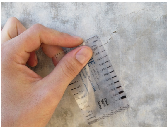
Figure A-72 - Shear crack (0.005 inches) (c in Figure A-69)
