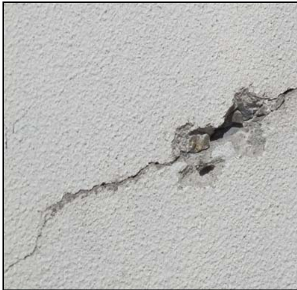
Figure A-47 - Spalling along main shear crack (b in Figure A-45)
