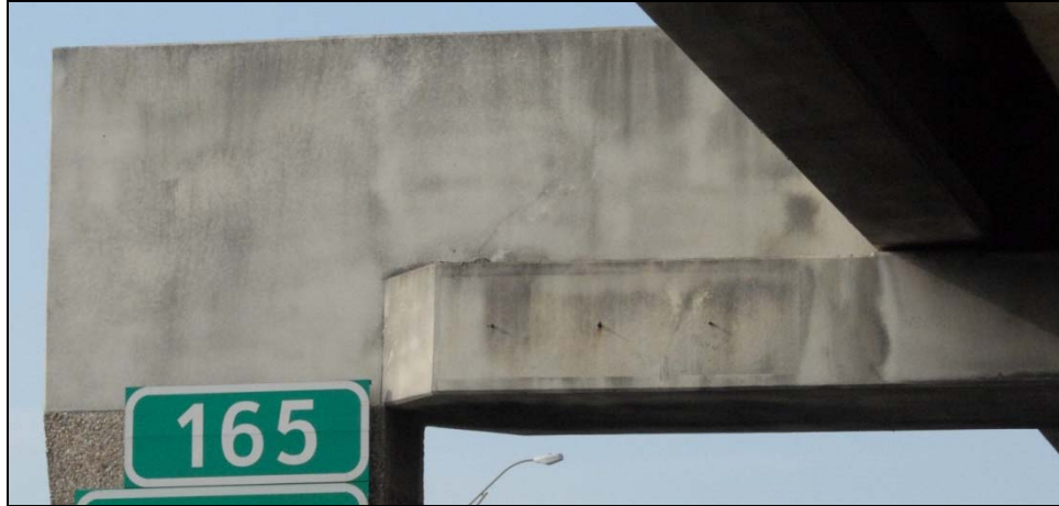
Figure A-31 - Overall view of NE corner of bent
