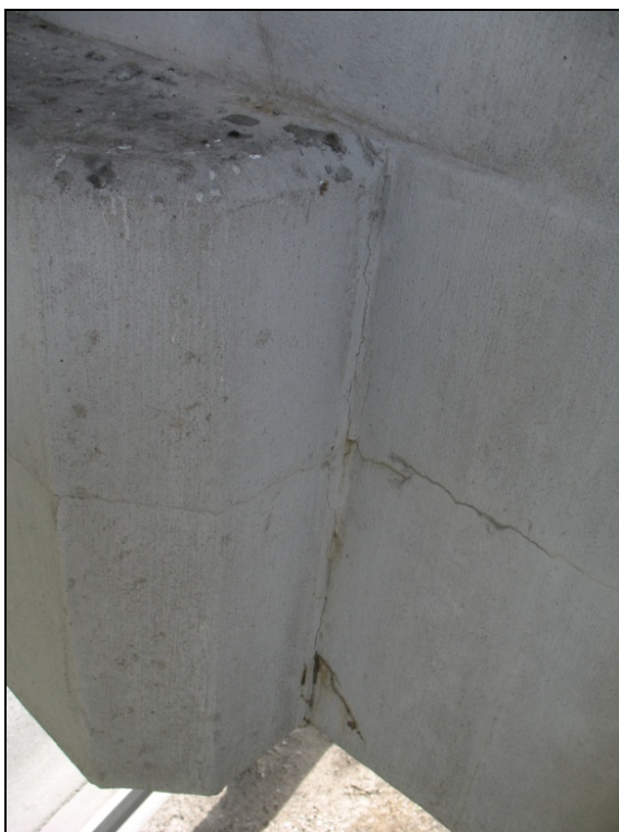
Figure A-14 - Web-ledge cracking (d in Figure A-10)
