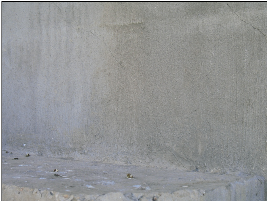
Figure A-7 – Small crack above ledge (b in Figure A-5)
