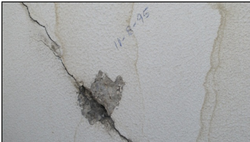
Figure A-42 – Spalling located along main shear crack (c in Figure A-39)
