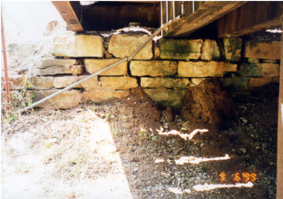
Photograph A.35: Deteriorated abutment at south end of south approach span
