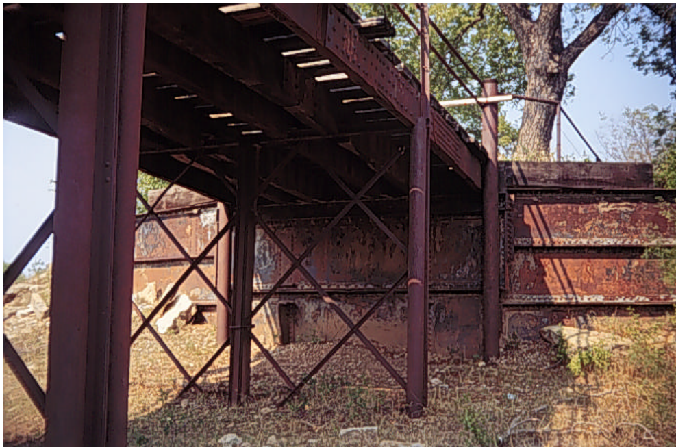
Photograph A.37: Details of the metal retaining wall at the north abutment
