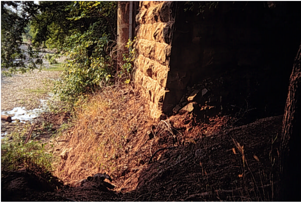
Photograph A.30: Details of the ground slope at the base of the south pier
