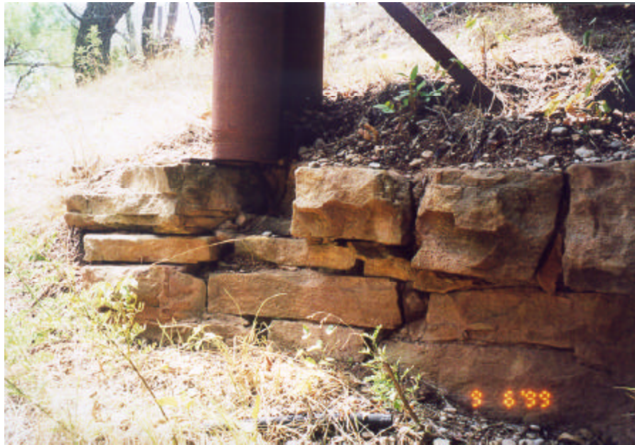
Photograph A.32: Details at base of pipe column of metal bent for north approach span
