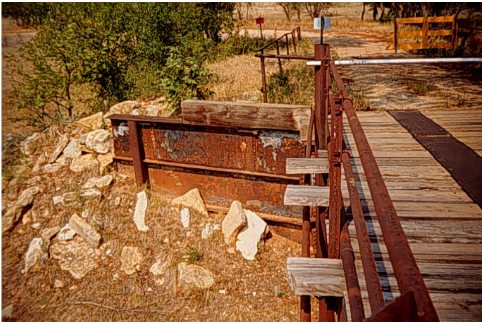
Photograph A.31: Details of the metal wing wall at the north abutment
