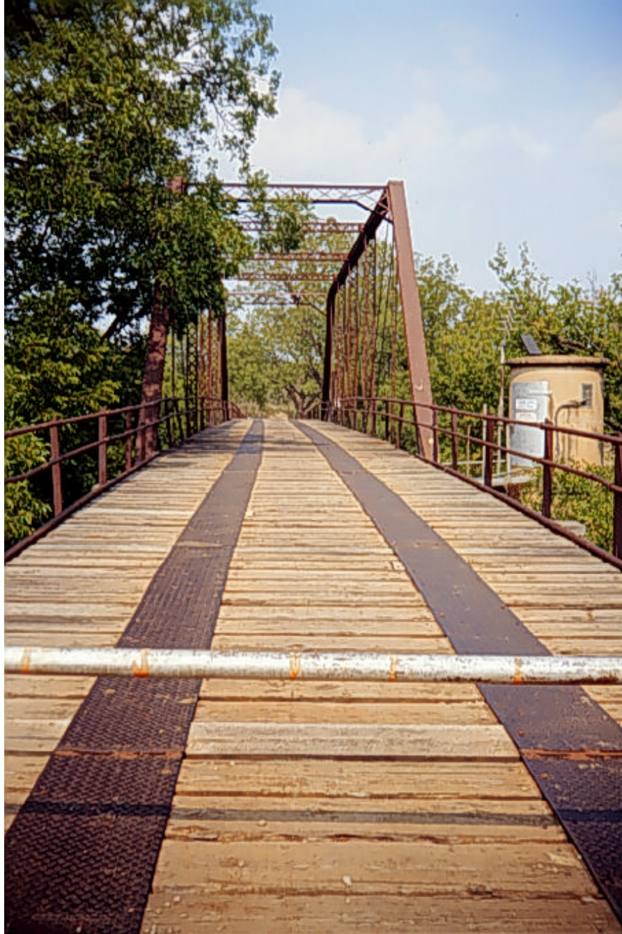
Photograph A.25: Details of the timber deck of the south approach span
