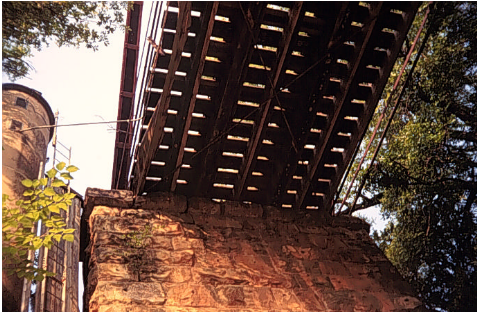
Photograph A.29: Details of the timber stringers of the main span resting on the south pier
