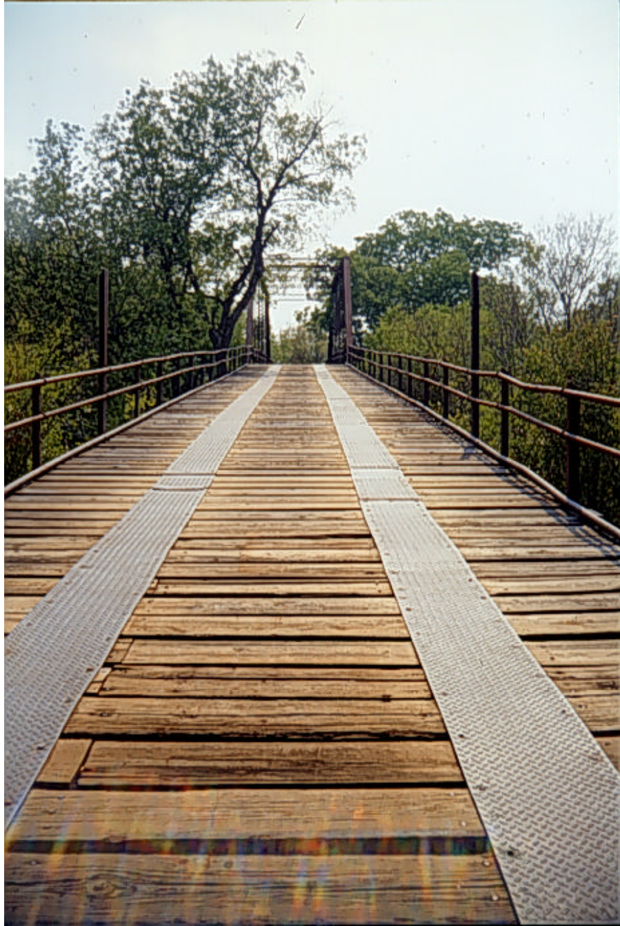
Photograph A.27: Details of the timber deck of the north approach span
