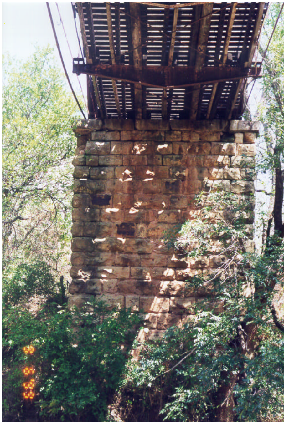
Photograph A.19: Details of the north stone masonry pier and the main span deck
