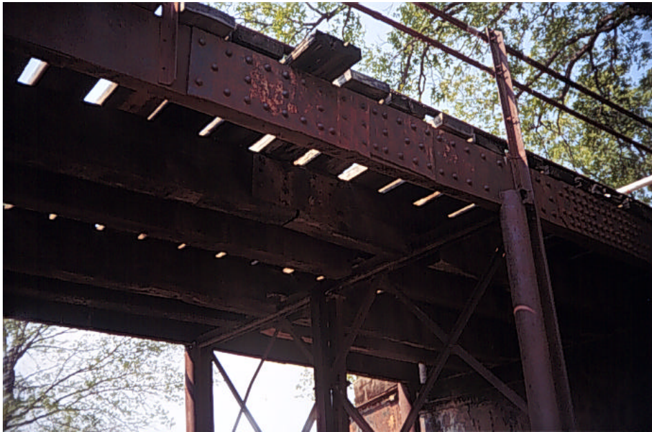
Photograph A.28: Details of the connection between timber stringers in the north approach span
