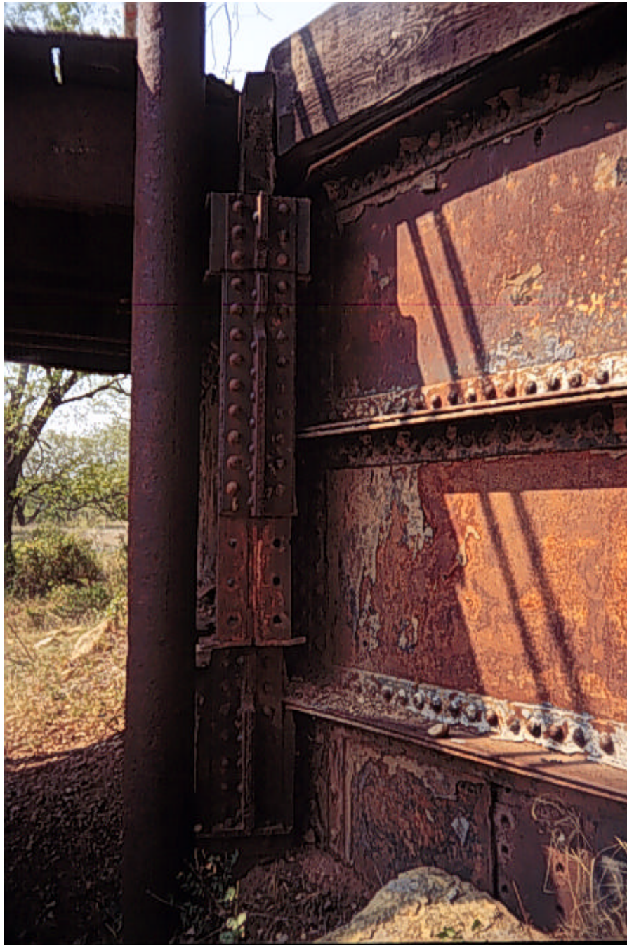
Photograph A.38: Details of the metal retaining wall at the north abutment
