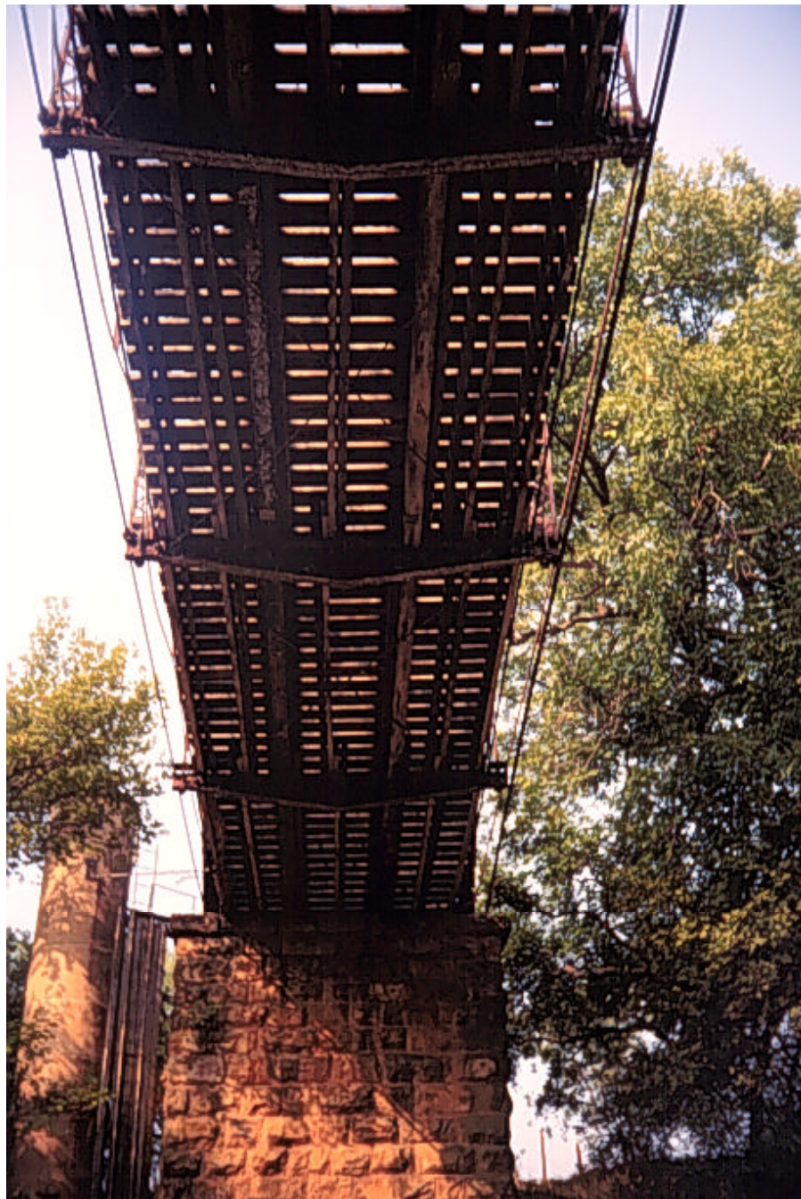
Photograph A.20: Details of the south stone masonry pier and the main span deck
