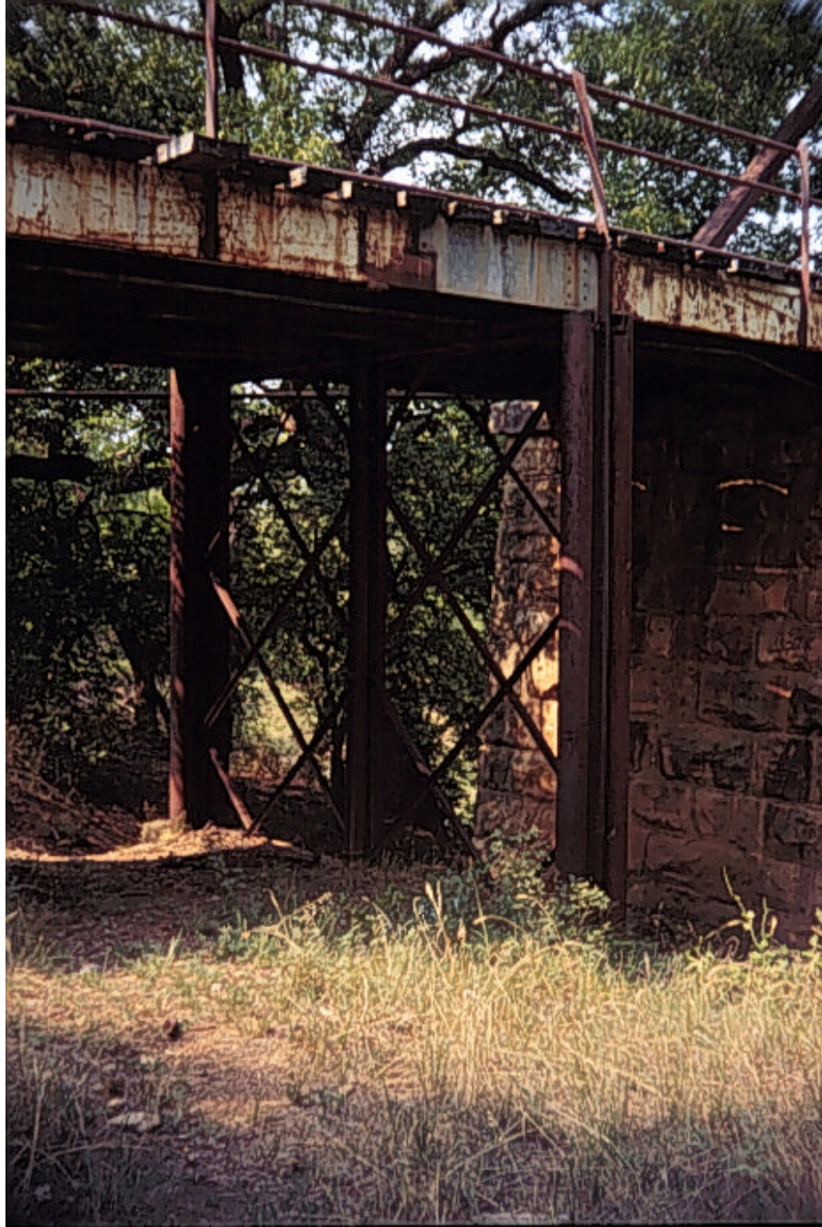
Photograph A.26: Details of the metal bent of the south approach span
