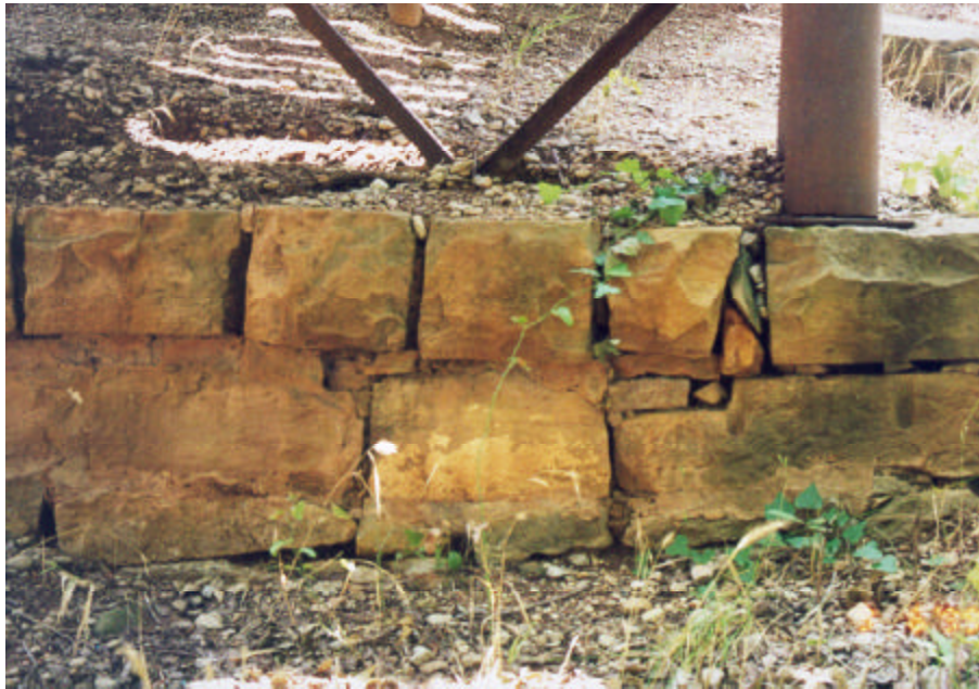
Photograph A.34: Deteriorated foundation of metal bents for north approach span
