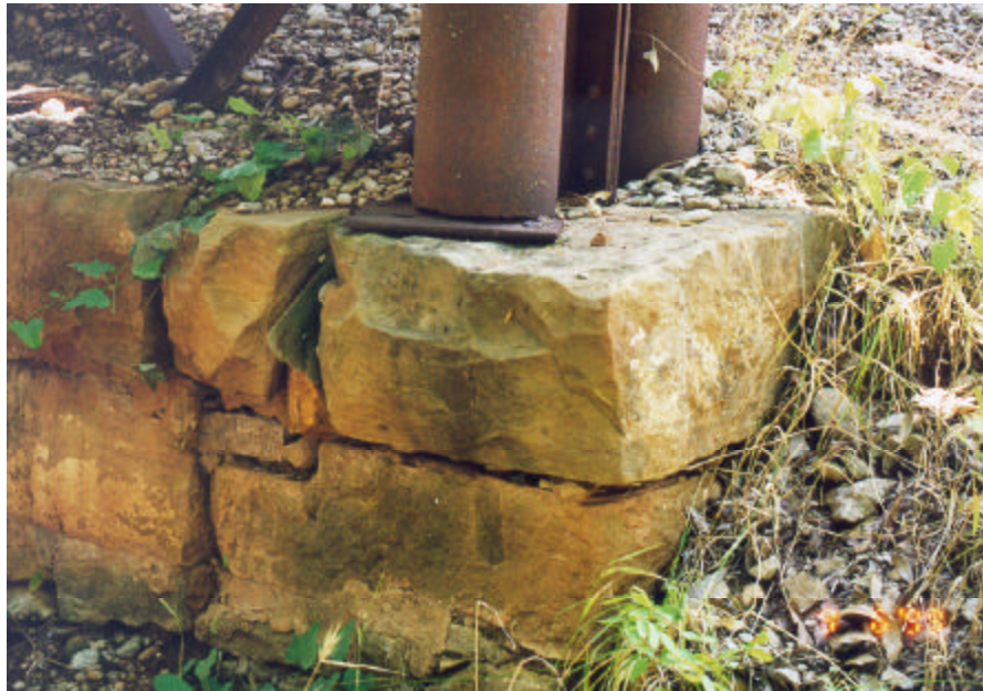
Photograph A.33: Details of base of pipe column of metal bent for north approach span
