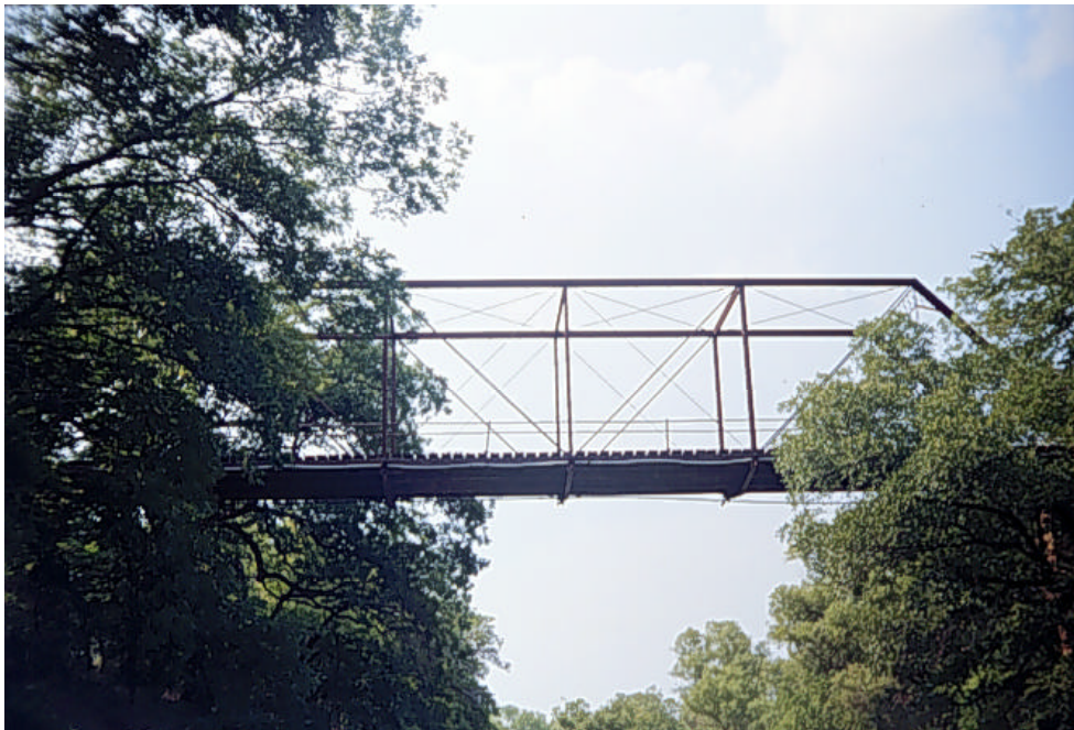
Photograph A.3: Side view of the main truss span of the bridge
