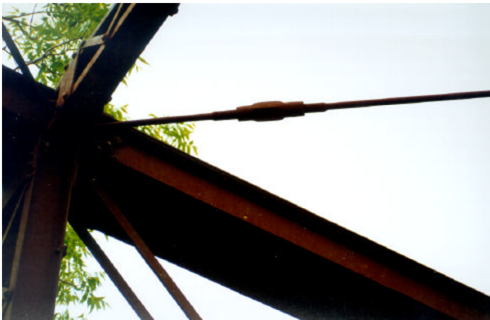
Photograph A.22: Details of the turnbuckle of the top bracing tension rods
