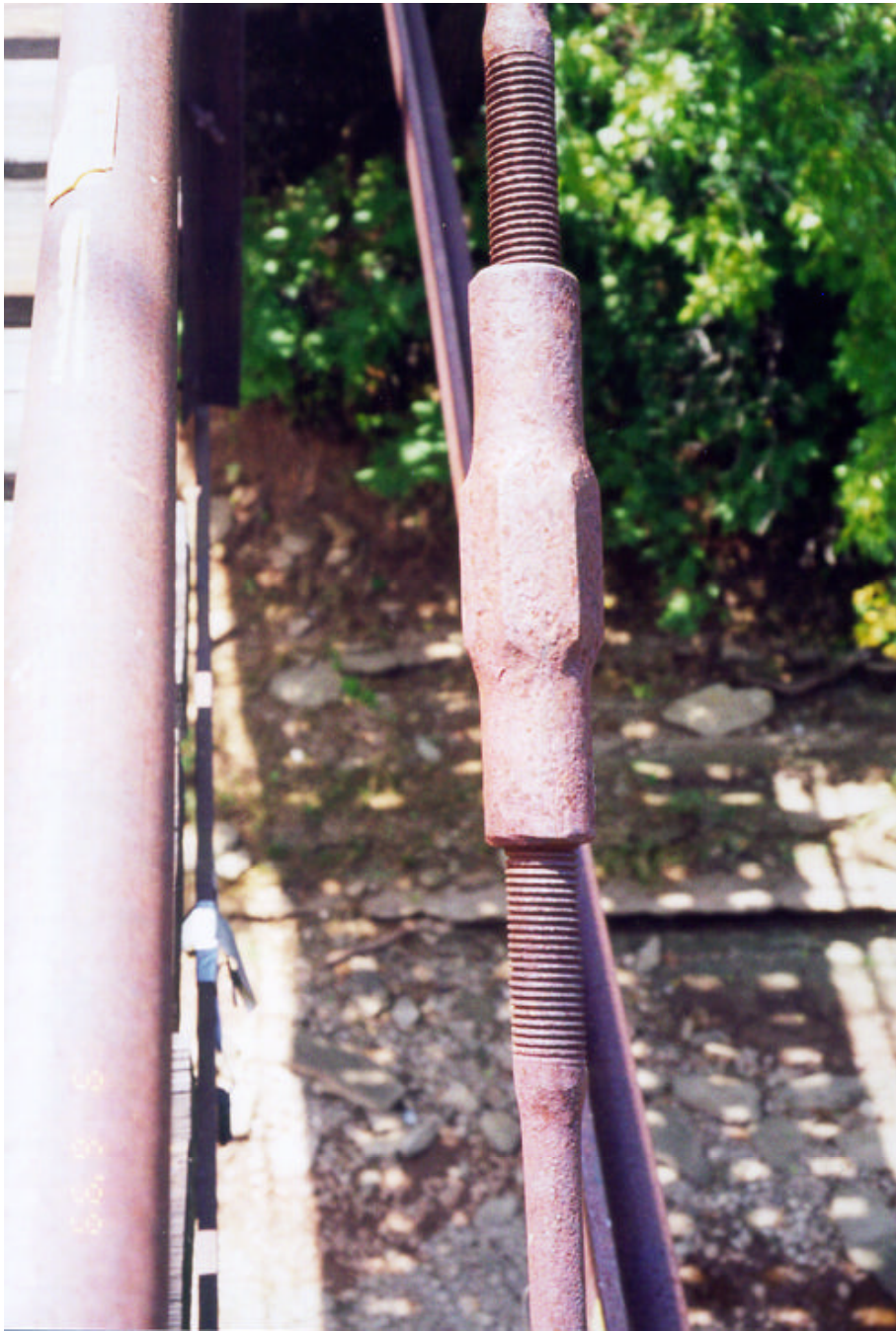
Photograph A.13: Details of tension rod L2U3 and L4U3, turnbuckle connection
