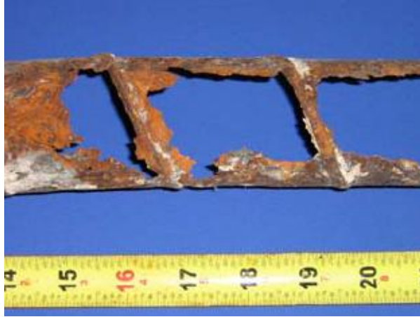
Figure 1.3: Corroded Hot Dip Galvanized Duct 22
