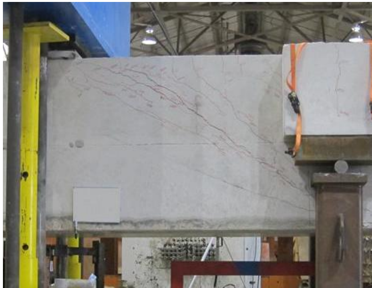
Figure D-39: Specimen after failure
