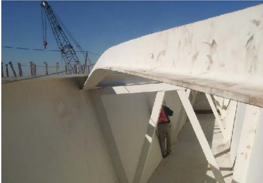
Figure 1.7: Trapezoidal Box Girder Failure During Construction
