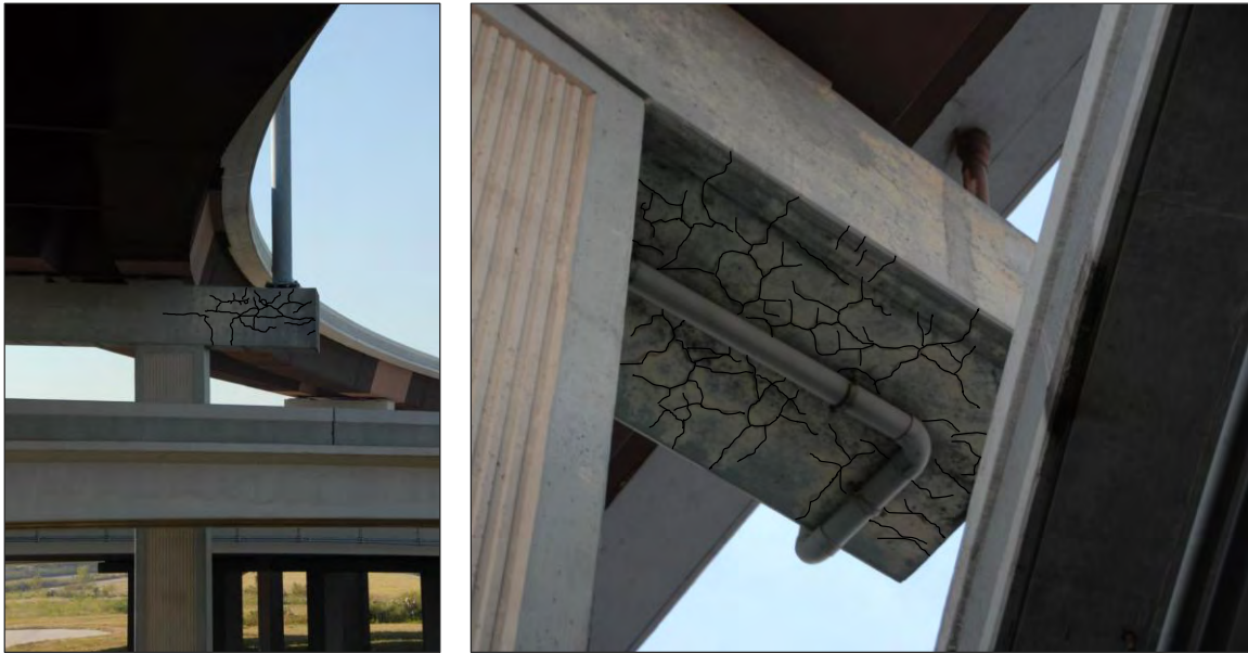
Figure 6-2: Signs of Deterioration within Connection Ramp Structures
