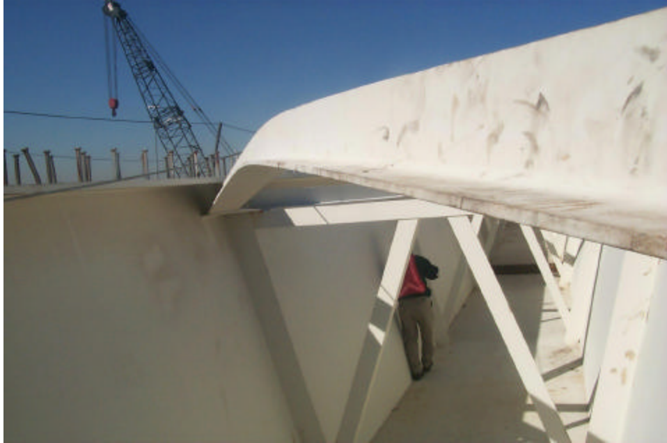
FIGURE 1.4 FAILURE OF TOP-LATERAL BRACE DURING BRIDGE ERECTION
