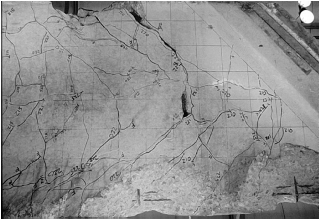
Figure D8: Photograph after Testing of Beam Underside, Box Beam 5 - Test 2
