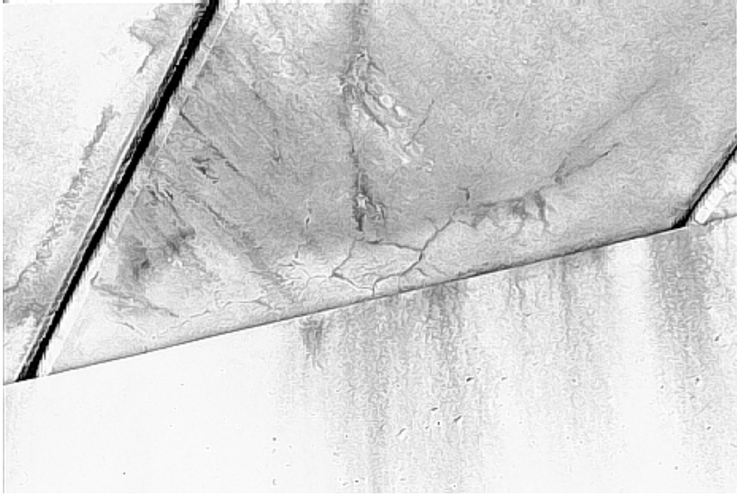
Figure 1.1: Cracking in bottom flange of box girder near support
