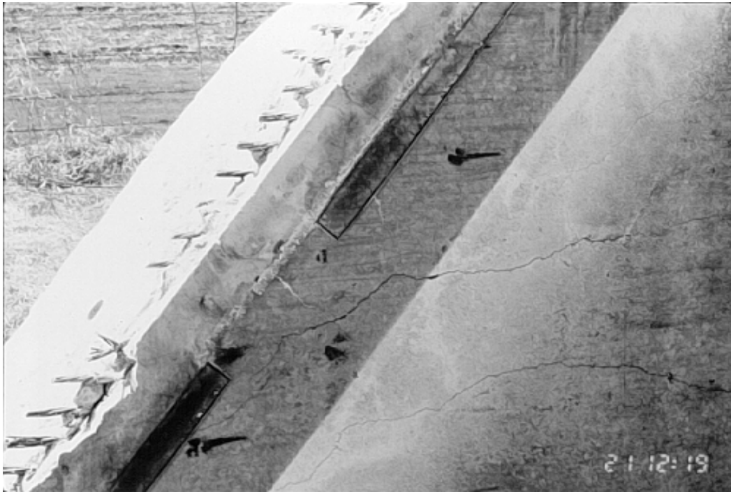
Figure 3.16: Cracking of 85-foot Box Beam used for Impact-Echo Testing
