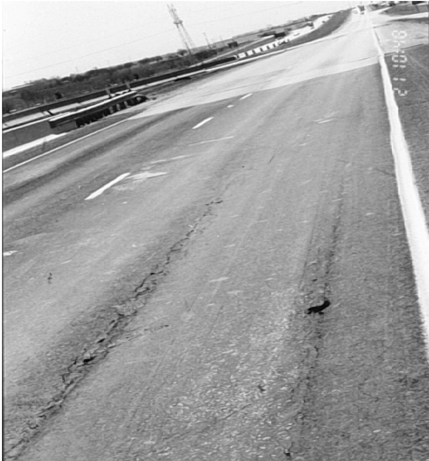
Figure 4.2: Longitudinal Cracks in Wearing Surface of Bridge Deck
