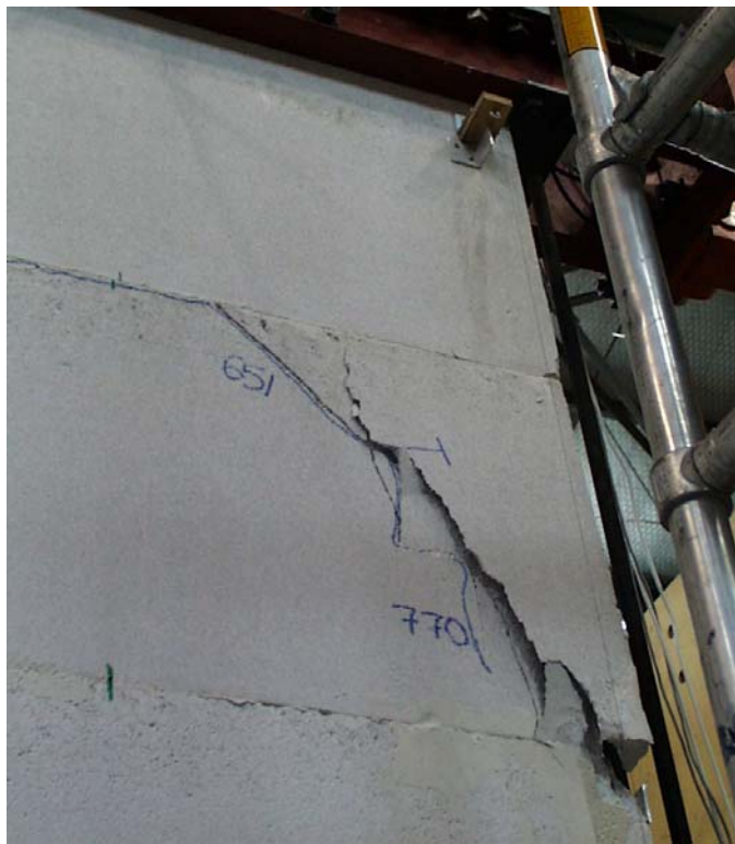
Figure 5-18: Cracked and spalled AAC at south end of Shear Wall Pilot Specimen 2 at end of test
