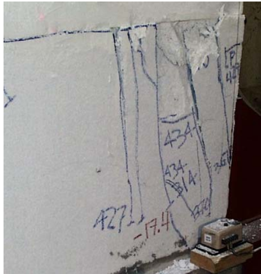
Figure 4-12: Cracks and spalled concrete at south end of Shear Wall Pilot Specimen 1 at end of test
