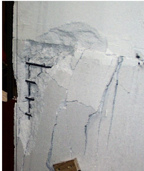
Figure 4-13: Back face of compression toe at end of test, Shear Wall Pilot Specimen 1
