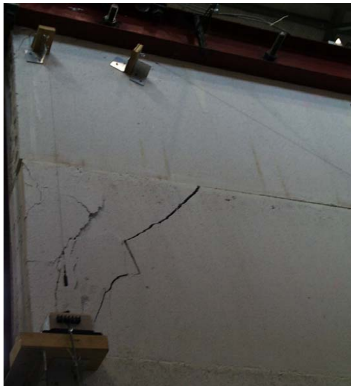
Figure 5-17: Cracked and spalled AAC on back of south end of Shear Wall Pilot Specimen 2 at end of test
