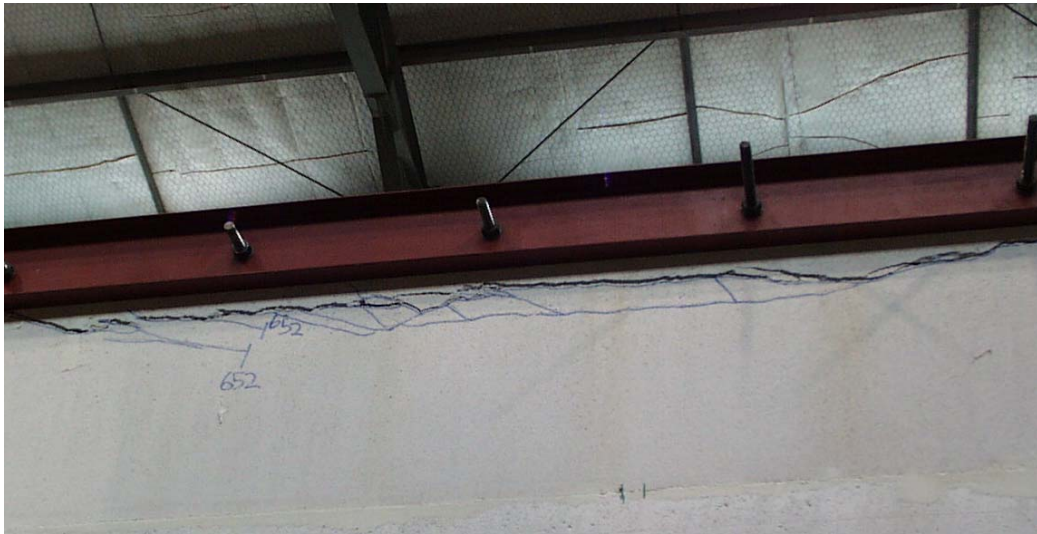
Figure 6-9: Tensile crack below bond beam
