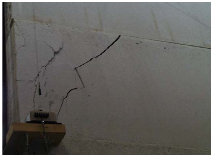
Figure 6-6: Crack on back of south end of Shear Wall Pilot Specimen 2 showing rotation of end of panel
