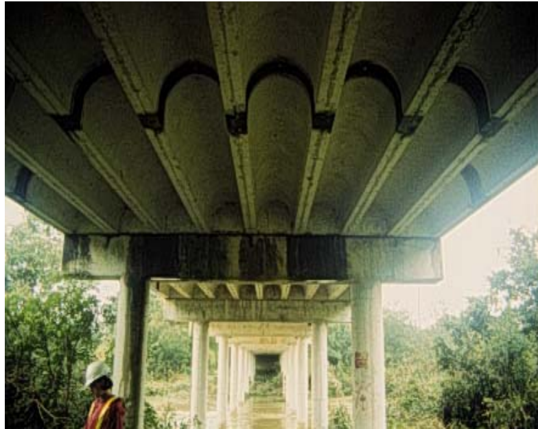
Figure 4.2 Photograph of Pan-Joist Bridge in Buda, Texas Indicating Uneven Surfaces on Bottom of Joists
