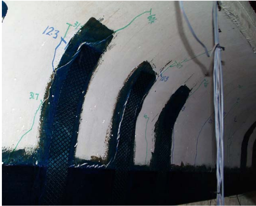
Figure 5.11 Initiation of Debonding Along CFRP Sheet
