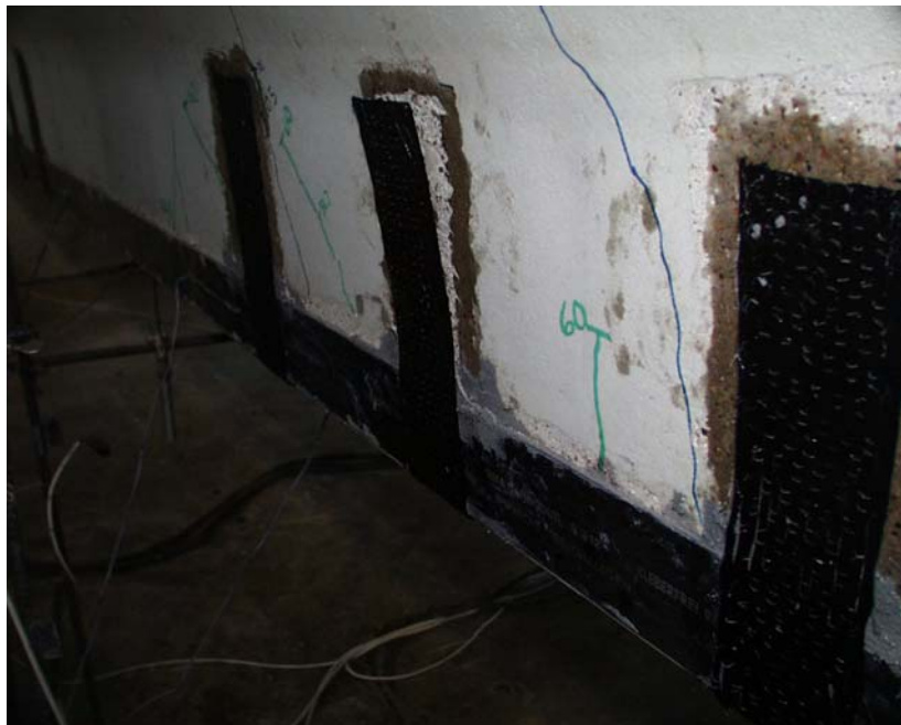
Figure 5.7 Transverse Strap Debonding at Ultimate Design Load
