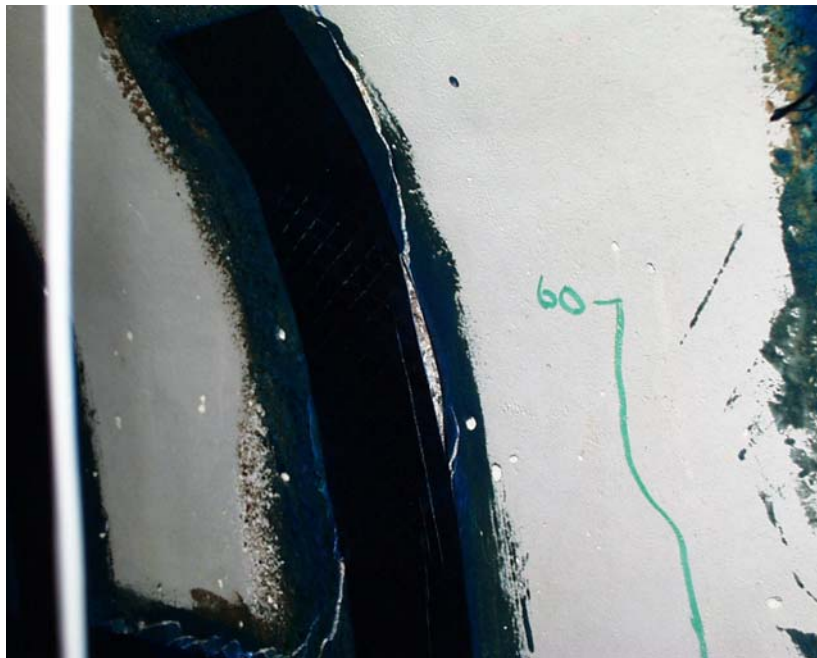
Figure 5.12 Crack Propagation Behind Strap Caused Debonding
