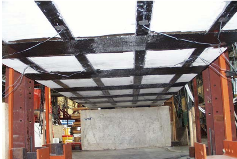
Figure 7.8 Picture of the Bottom Surface of Specimen FS-1 after Strengthening with the CFRP Pultruded System
