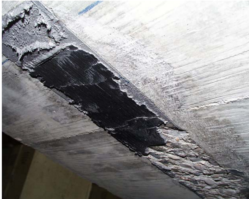
Figure 8.9 Evidence of Plate Delamination of the East CFRP Plate at the North End of Specimen FS-1
