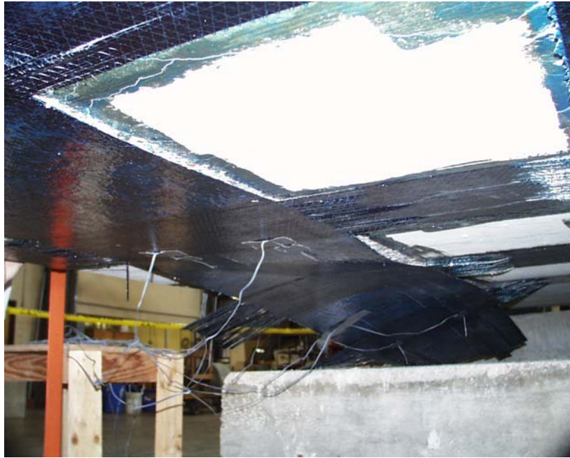
Figure 8.13 View of West CFRP Sheet after Debonding from Specimen FS-2
