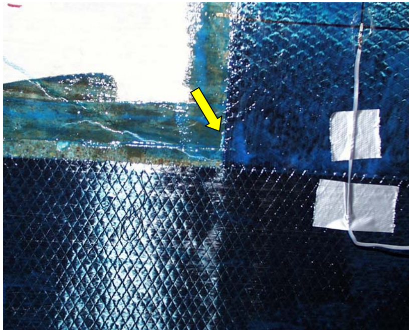
Figure 8.12 Initiation of Debonding Along CFRP Sheet
