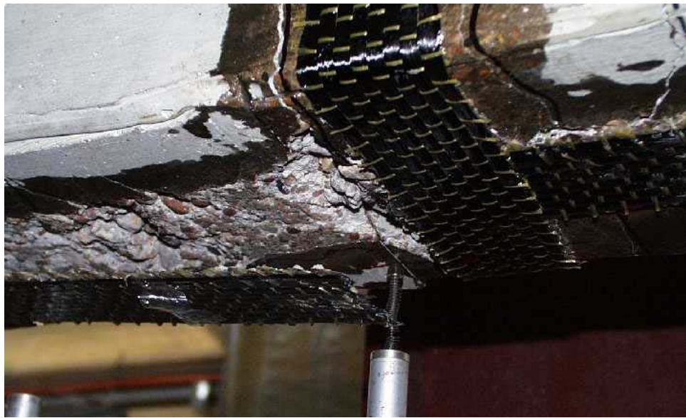
Figure 4.11: Rupture of Composite at Critical Section
