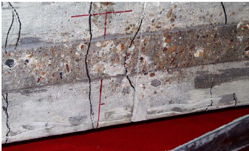
Figure 4.18: Evidence of Poor Composite Bond
