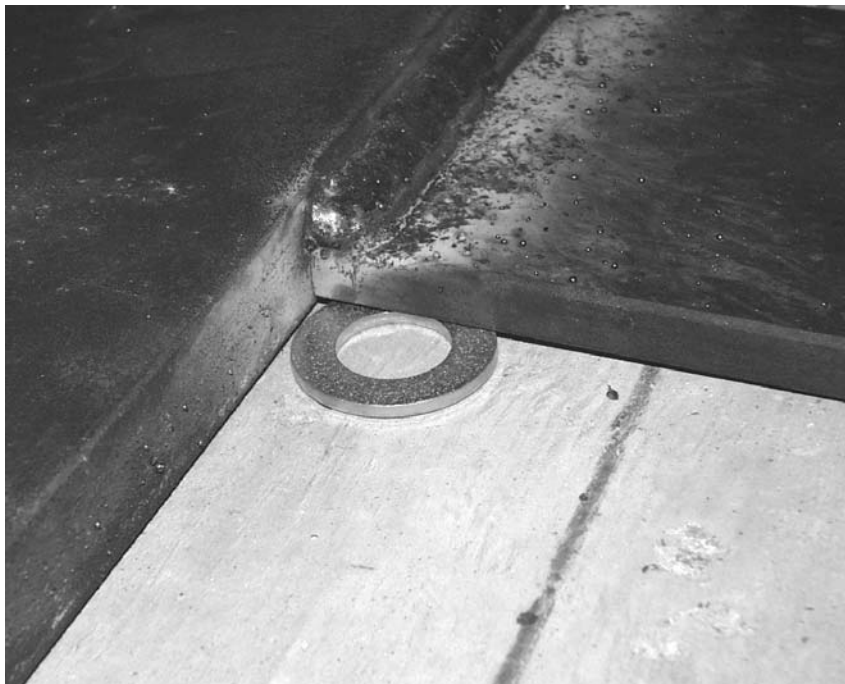
Figure 6.7: Gap between small plate and concrete slab
