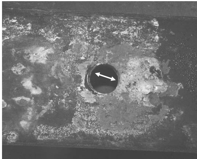
Figure 6.28: Slight steel plate deformation of MAXIB01
