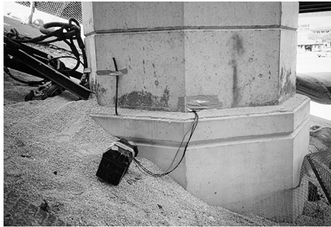
Figure 4.14: Cast-in-place base forming a rigid moment connection between base segment PC16-1 and foundation.
