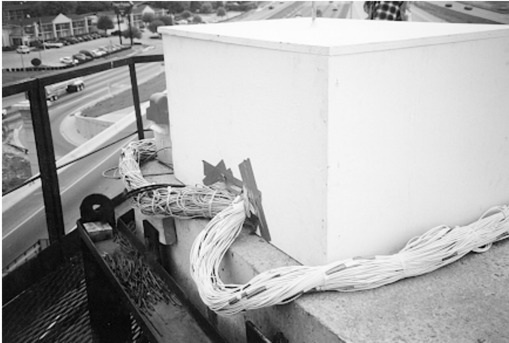
Figure 3.29: Data recording equipment in place at top of pier.
