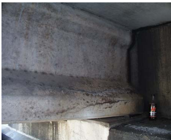
Figure 7.6 View of greater damage to SW Girder 2
