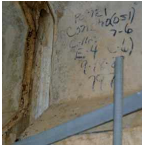
Figure 7.33 Horizontal and map cracking at girder ends (Bent 9)
