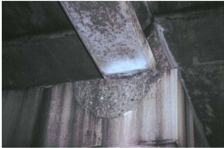
Figure 7.4 Missing bearing pad at I-10 structure
