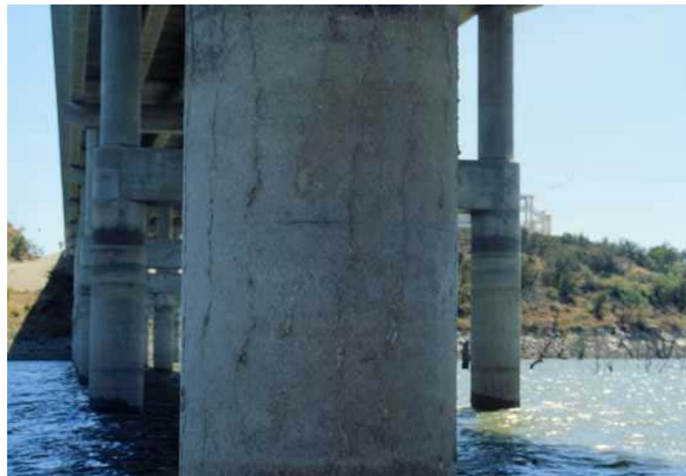
Figure 7.25 Horizontal and vertical cracking in Bent 5 of FM 1979 structure
