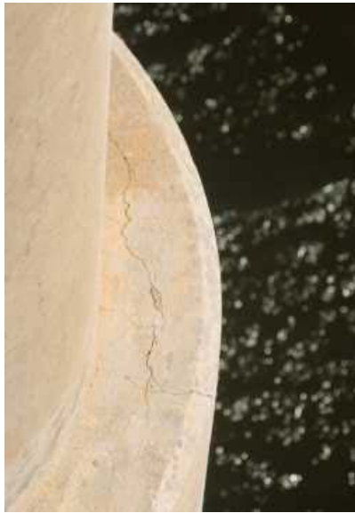
Figure 7.31 Propagation of vertical cracks in lower column to top of tie beam (Bent 5)
