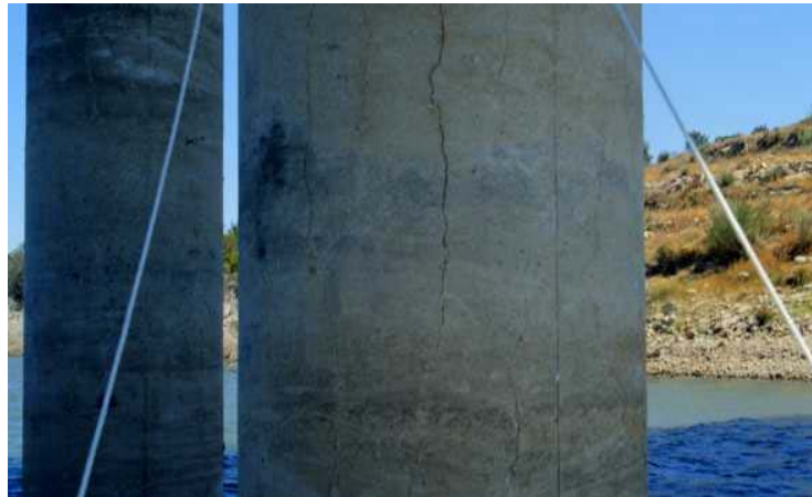
Figure 7.24 Vertical cracking typical of Bents 9, 10 and 11 of FM 1979 structure (Bent 10)
