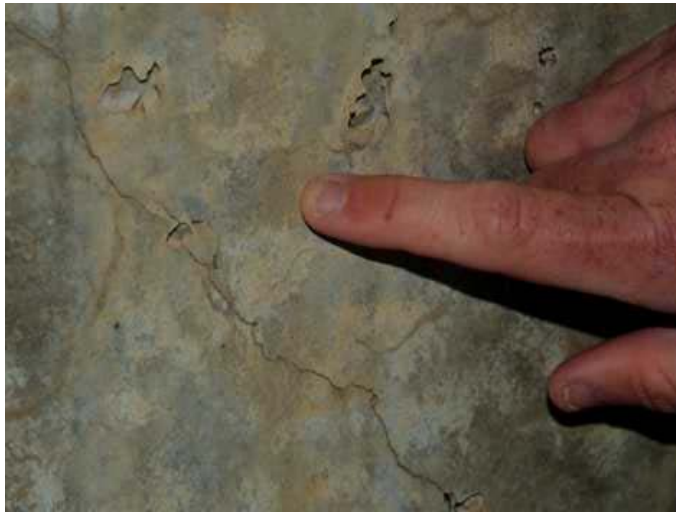
Figure 7.29 Map cracking on side of bent cap (Bent 5)
