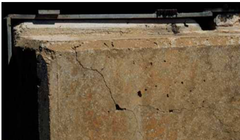
Figure 7.32 Map cracking at ends of bent cap (Bent 9)
