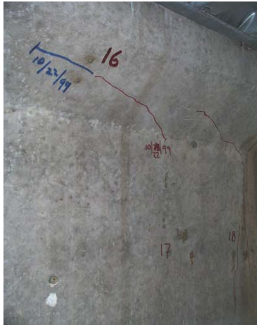
Figure 7.15 Extension of crack on Face 2 of NW Girder 3 at Robinson Road structure
