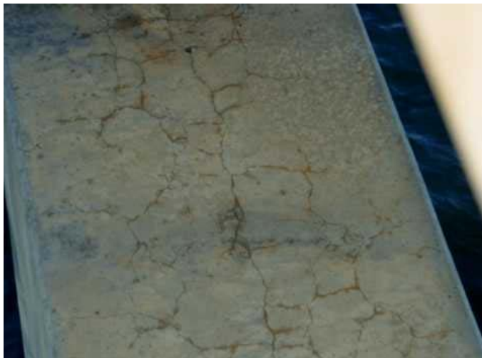
Figure 7.30 Map cracking on upper surface of tie beam (Bent 5)
