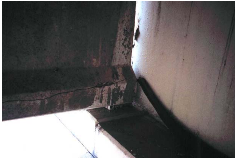
Figure 7.11 Rubber seal dropped from joint above at west abutment of US-90 structure
