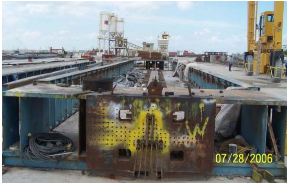
Figure 3-9: Prestressing bed at HEI Corpus Christi Plant (photograph courtesy of Chris Leonard)
