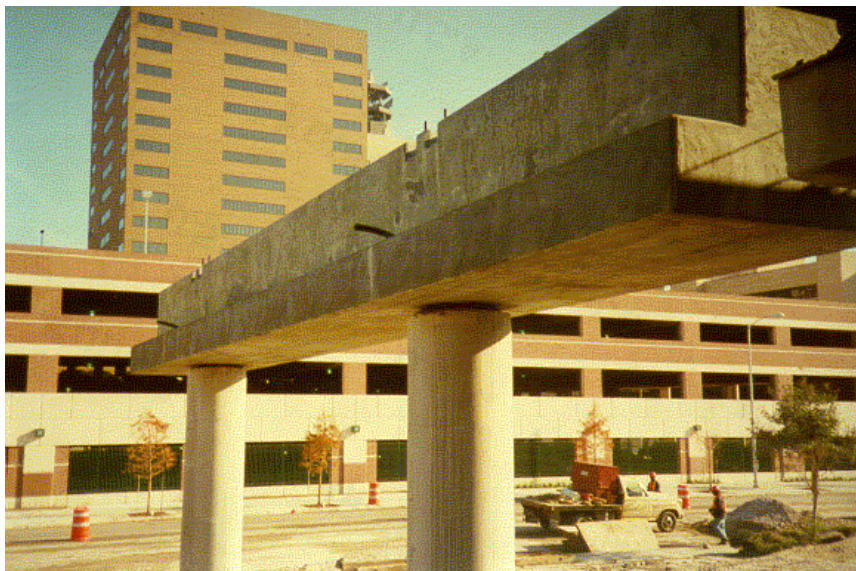
Figure 1.10 Precast Bent Cap Resting on Shims prior to Grouting of Bedding Layer and Sheathing Ducts
