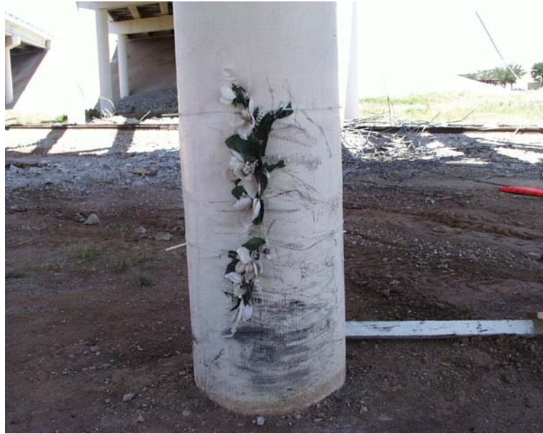
Figure 7.7 Vehicular collision damage on column of Structure #2.
