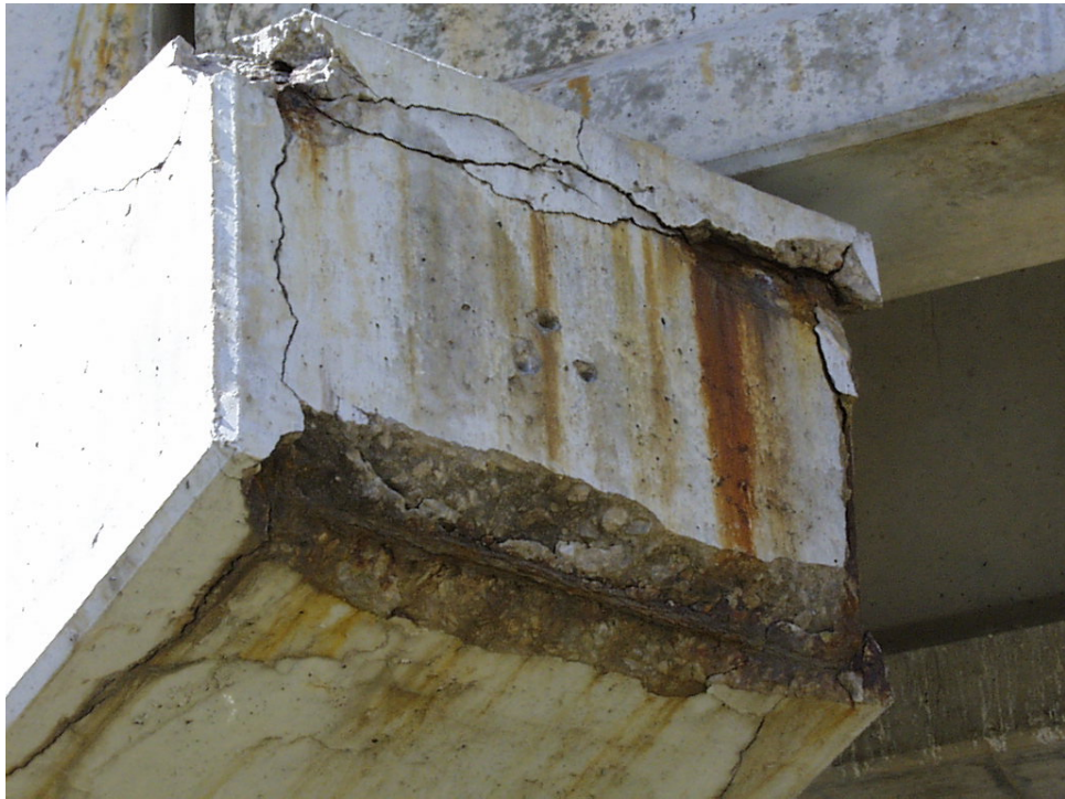
Figure 5.8 Damage to an endcap of Structure #5.
