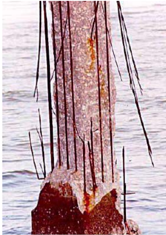
Figure 3.3 Concrete pile that had previously been repaired with a fiberglass jacket.
