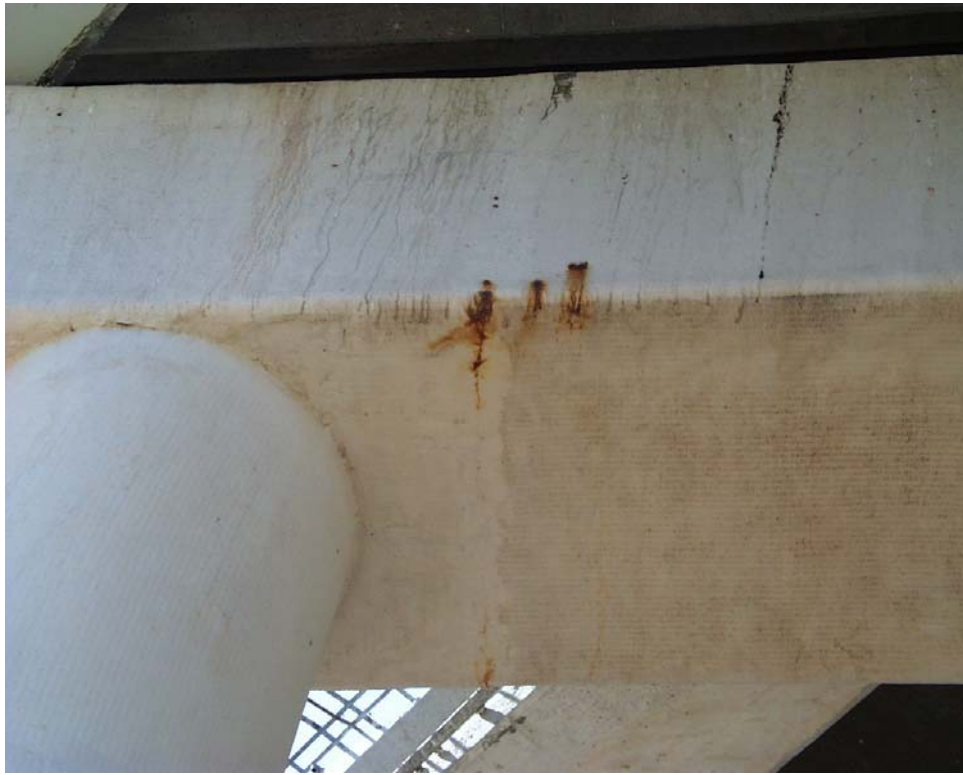
Figure 5.8 Rust stains on bent of Structure #1.
