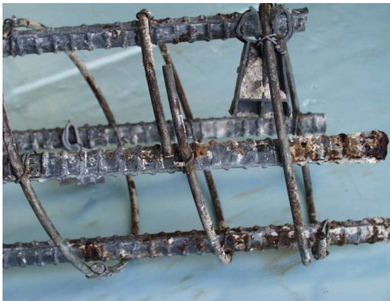
Figure 6.17 Steel reinforcing of CC6 with a corrosion rate of 1.41 mpy.
