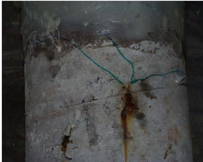
Figure 6.10 Evidence of corrosion activity in the splash zone of specimen CNC10.
