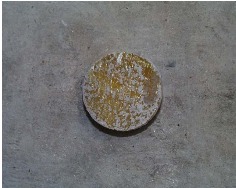
Figure 6.12 Failure at the epoxy/concrete interface on Test #2.
