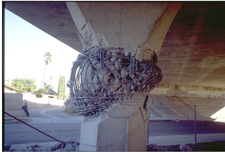
Figure 3.2 Highway bridge column after the 1994 Northridge earthquake (Courtesy of EERC, University of California, Berkeley).
