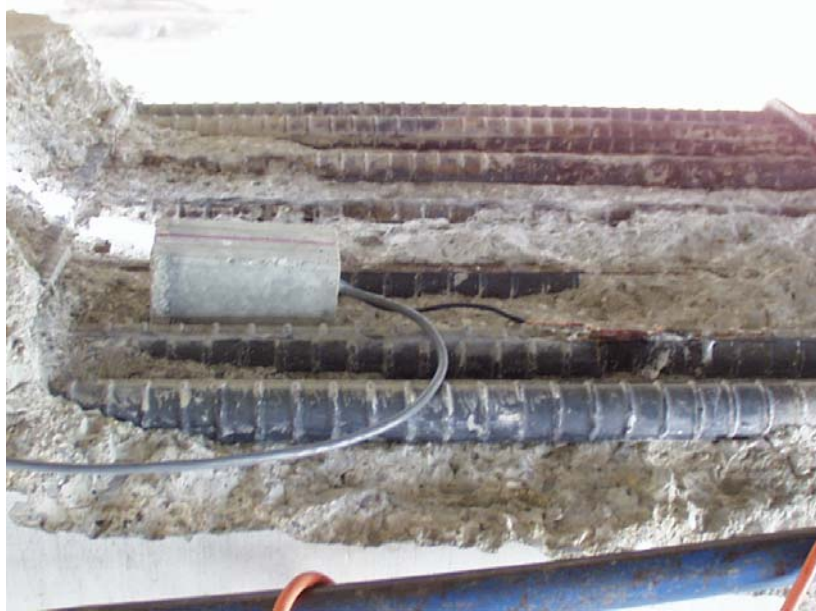
Figure 5.15 Installed probe on Structure #7.
