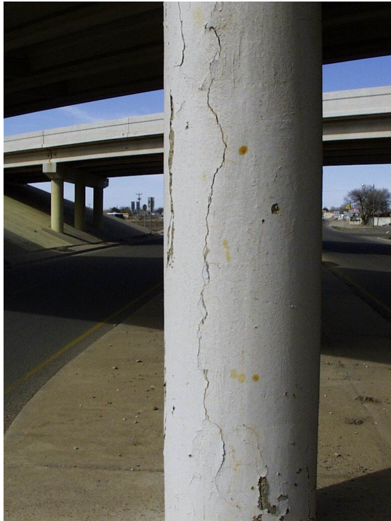
Figure 5.10 Cracking on column of Structure #12.
