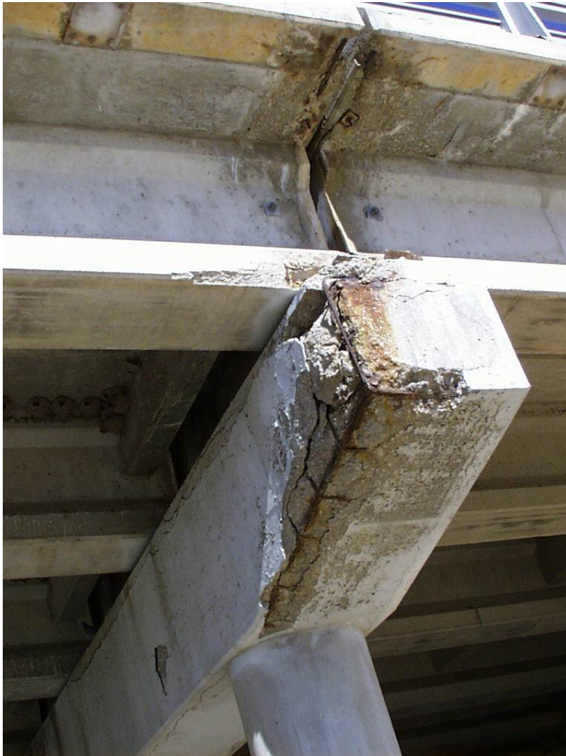
Figure 5.9 Delamination on an endcap of Structure #8.
