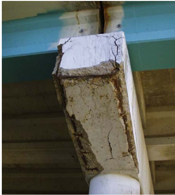
Figure 1.1 Corrosion damage to a bridge bent.
