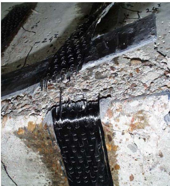
Figure 5.15.c: Debonding of the north end of the longitudinal plate and rupture of the transverse anchorage
