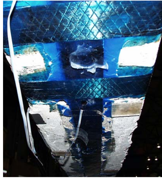
Figure 5.30.b: Debonding of longitudinal sheet (zoom Figure 5.30.a)
