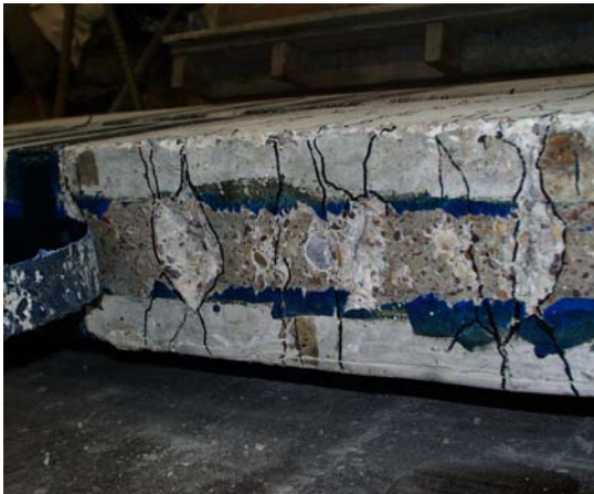
Figure 5.30.c: Sheet-concrete interface; concrete wedges pulled off at rupture; cracking in debonding initiation zone; few concrete pieces attached along the laminate
