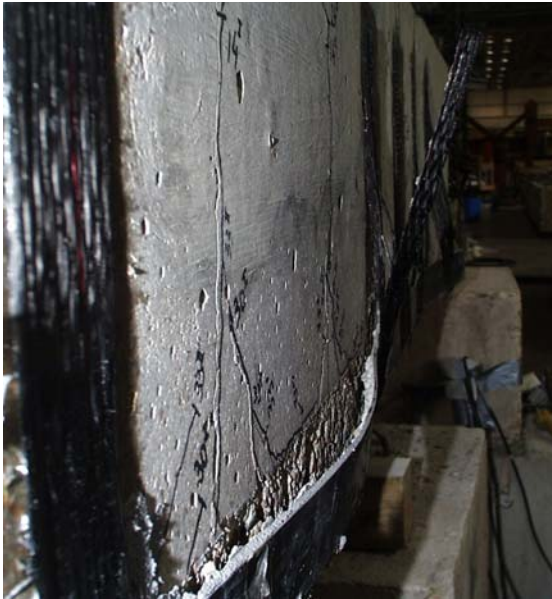
Figure 5.15.a: Debonding of the CFRP pultruded plate at midspan
