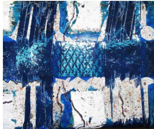
Figure 5.30.d: Transverse anchorage pulled off by debonding and slipping of longitudinal sheet; smooth concrete surface under longitudinal laminate
