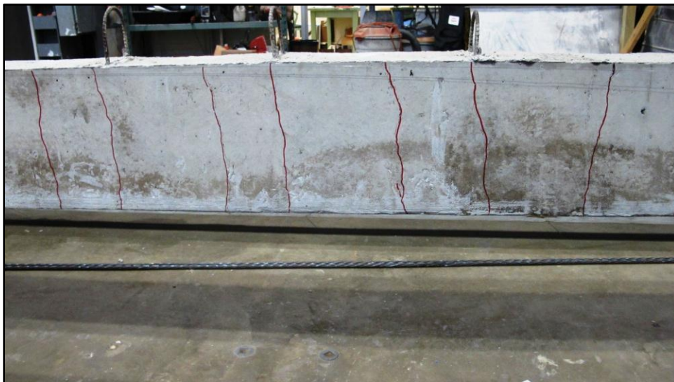
Figure 5-19: Cracking in SP1 after Buckling Failure (Test SP1-PT0-EX-2)
