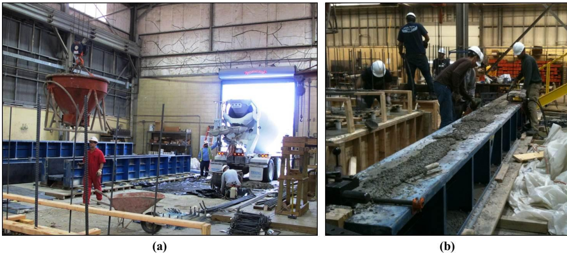
Figure 3-6: Specimen Casting; (a) Concrete transport from truck to formwork via crane bucket; (b) Consolidation via internal vibration
