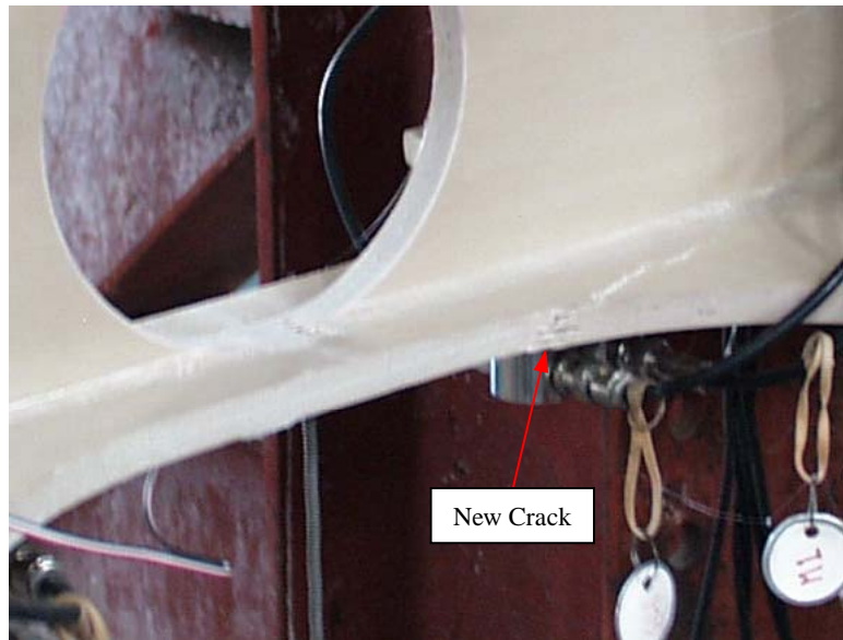
Figure 4.45: Additional Crack at Bottom Flange
