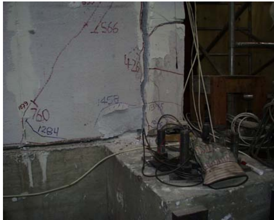
Figure A.35 Loss of end block on compression toe in Shear Wall Specimen 16
