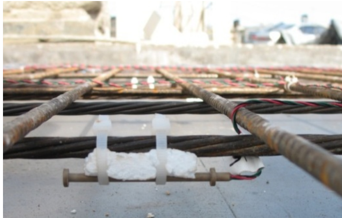
Figure 4.9 Embedment gage installed parallel to a prestressing strand (Foreman 2010)
