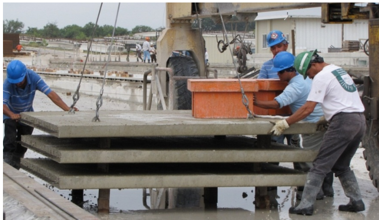
Figure 4.18 Panels being lifted out of prestressing bed and stacked at Plant A
