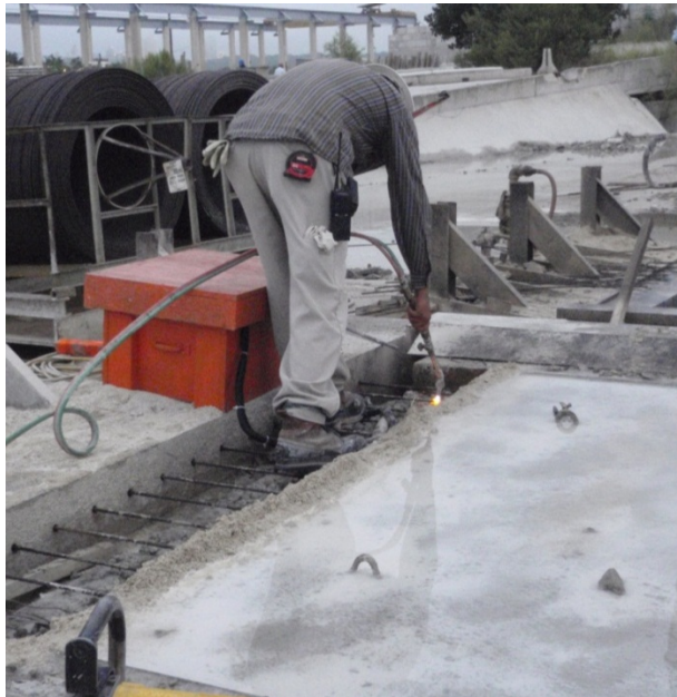
Figure 4.16 End strands being torch-cut at Plant A
