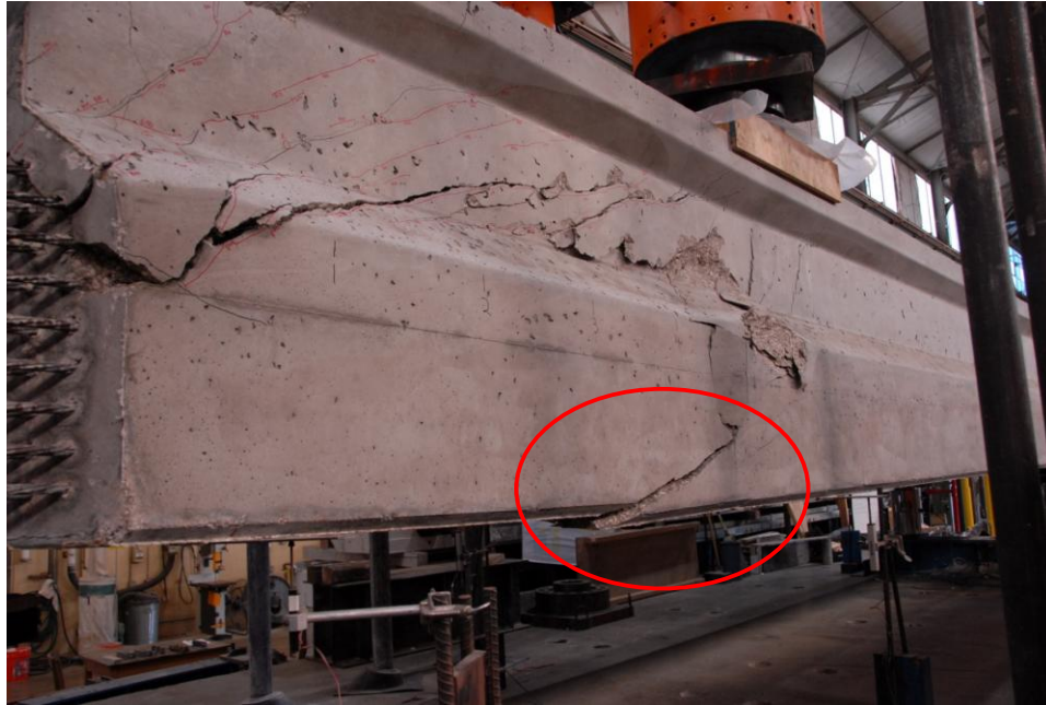
Figure 6-29: Shearing through bottom flange. Skewed end of 5B40-4 is shown.
