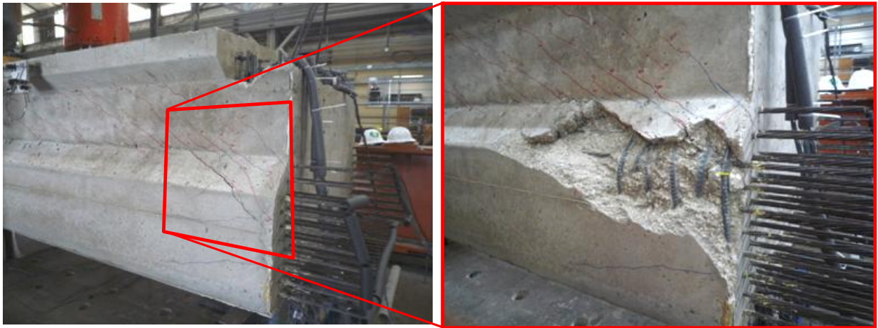
Figure 6-16: Spalling of cover at end of beam. Square end of 5B40-1 is shown.
