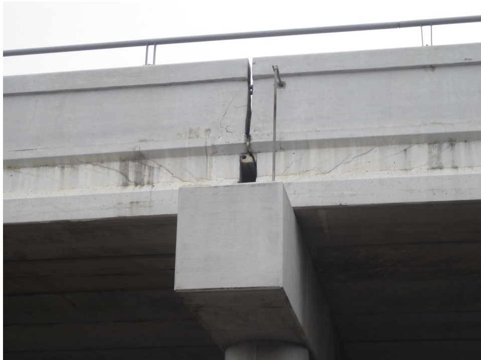
Figure 6-1: Diagonal cracks in box beams over central bent cap in bridge over IH35.
