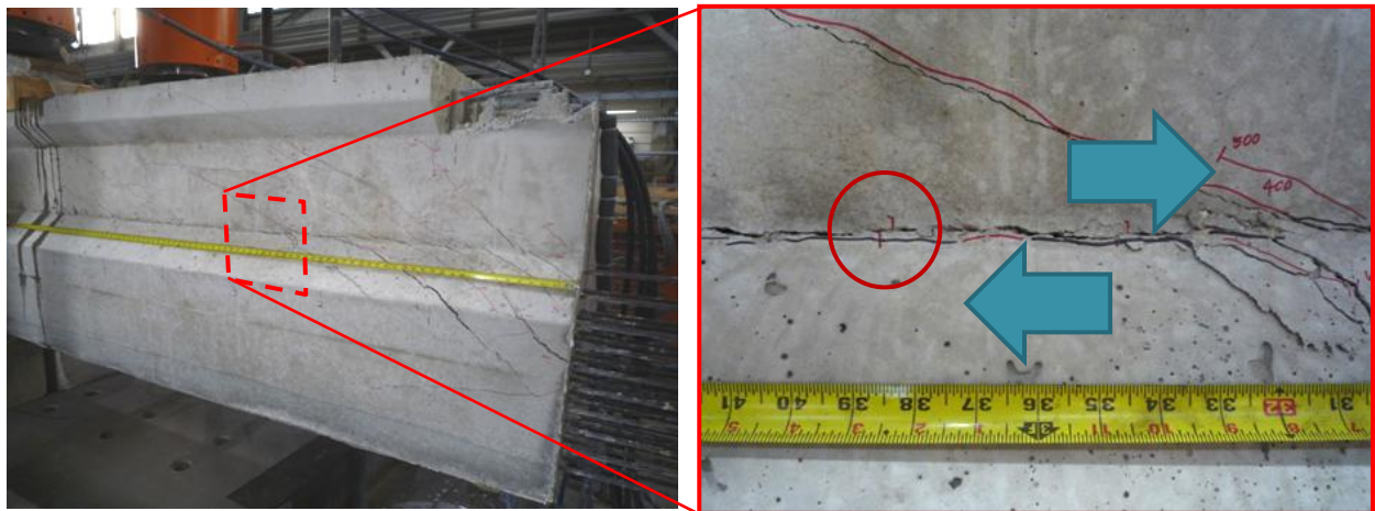
Figure 6-26: Signs of horizontal shear distress. Square end of 5B40-3 is shown.
