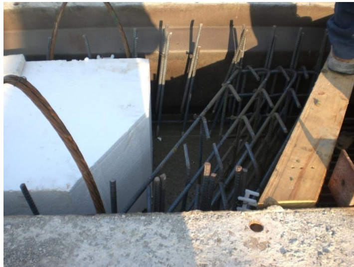
Figure 3-5: Hybrid void at 30° skewed end of 4B28 Box Beam.
