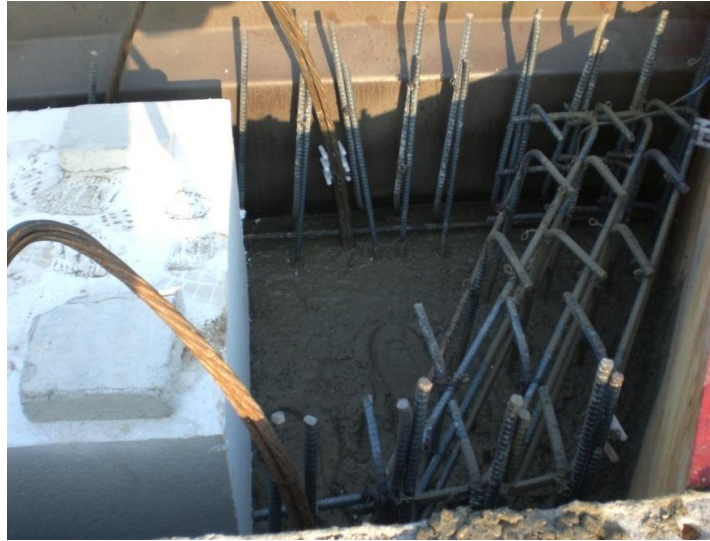
Figure 3-3: Square void at 30° skewed end of 4B28 Box Beam.
