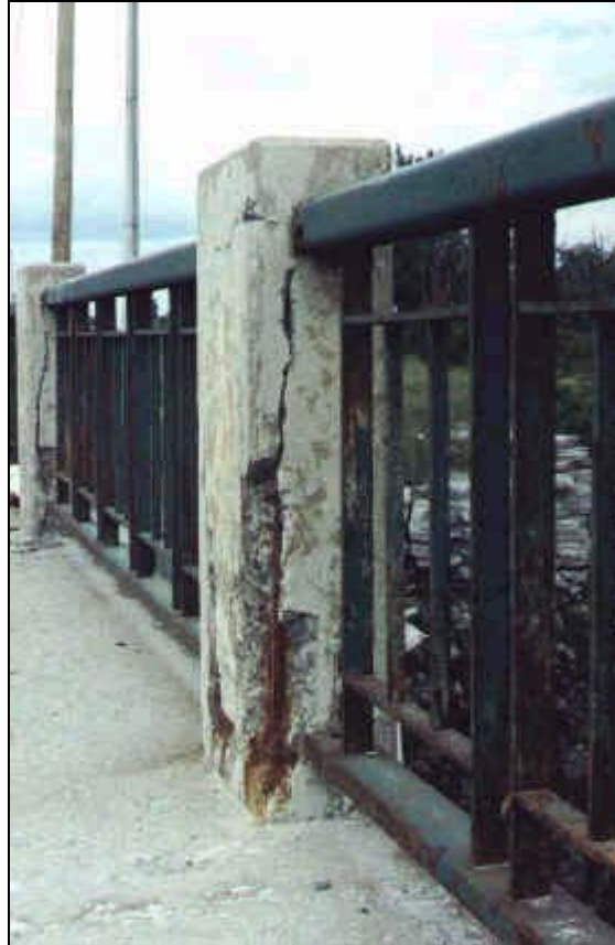
Figure 1.1 Concrete degradation caused by rebar corrosion damage near Kingston, Ontario (Roberge 1999)
