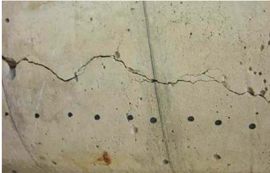
Figure 4.3 Large crack on lower surface of CC11 (Typical)
