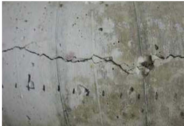
Figure 4.1 One of two large cracks located at upper-portion of CC10.
