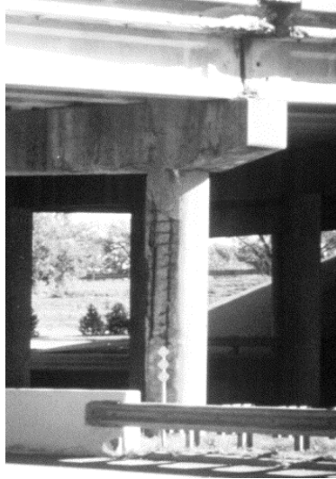
(a) Deicing Chemical Exposure "Attack from Above"
