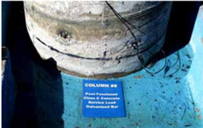
Figure 4.30 Condition of Specimen PT-TC-S-GB at the End of Testing 1
