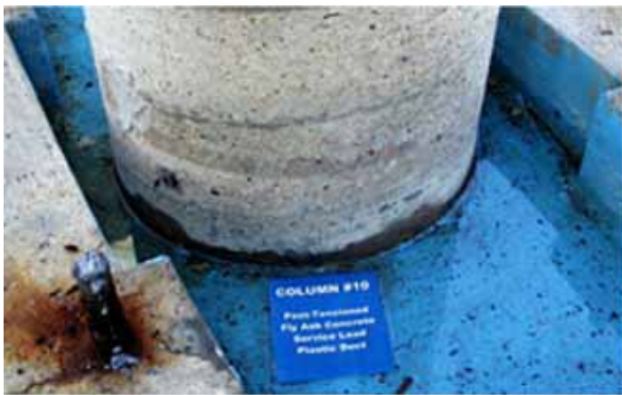
Figure 4.24 Condition of Specimen PT-FA-S-PD at the End of Testing 1
