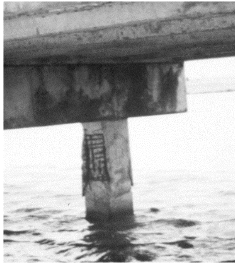
(b) Coastal Saltwater Exposure "Attack from Below"
