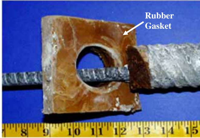
Figure 5.2 Duct Corrosion Found Inside Rubber Gaskets 1
