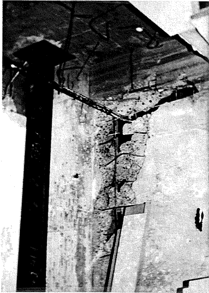
Figure 5- F7 Damage in concrete walls
