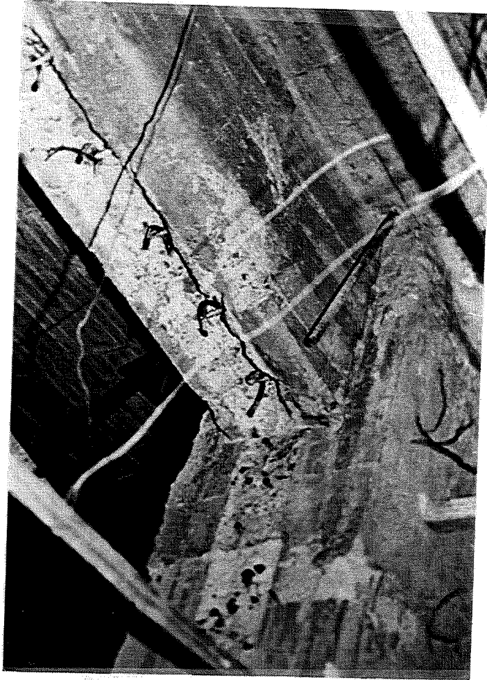
Figure 5- F9 Deficient wall-beam anchorages
