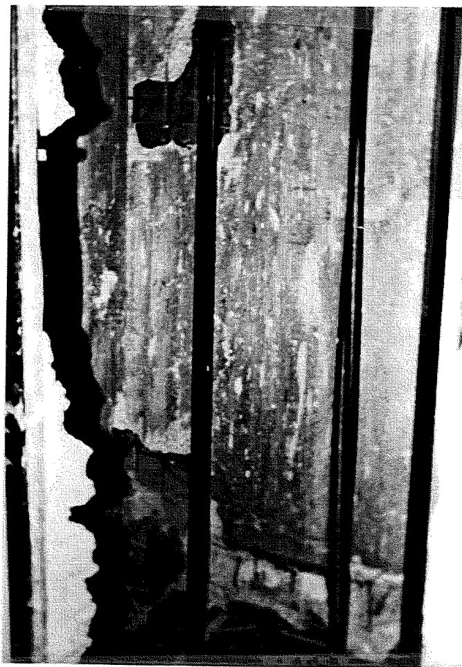
Figure 5- G5 Exposed reinforcement in concrete wall
