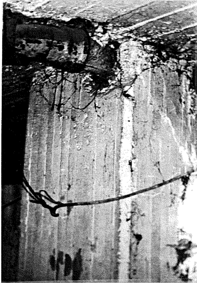
Figure 5- G4 Cracks in column at sewer pipe location
