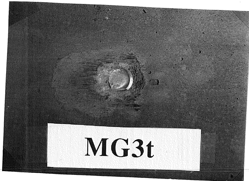
Figure 4.5 Frictional wear on grout surface.
