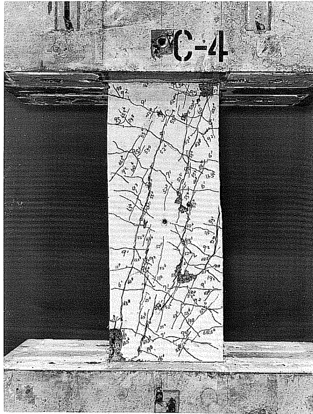
Fig. 11 Final Crack Pattern of Column Specimen
