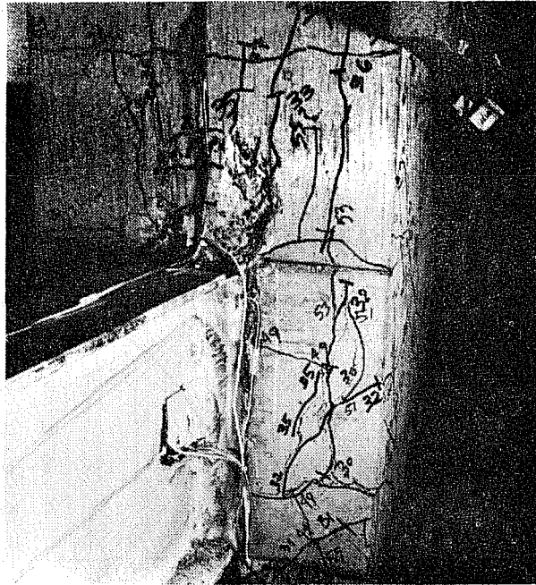
Fig. 4.8 A view of joint 2 after failure. (Top flange in compression in L1 and U1)
