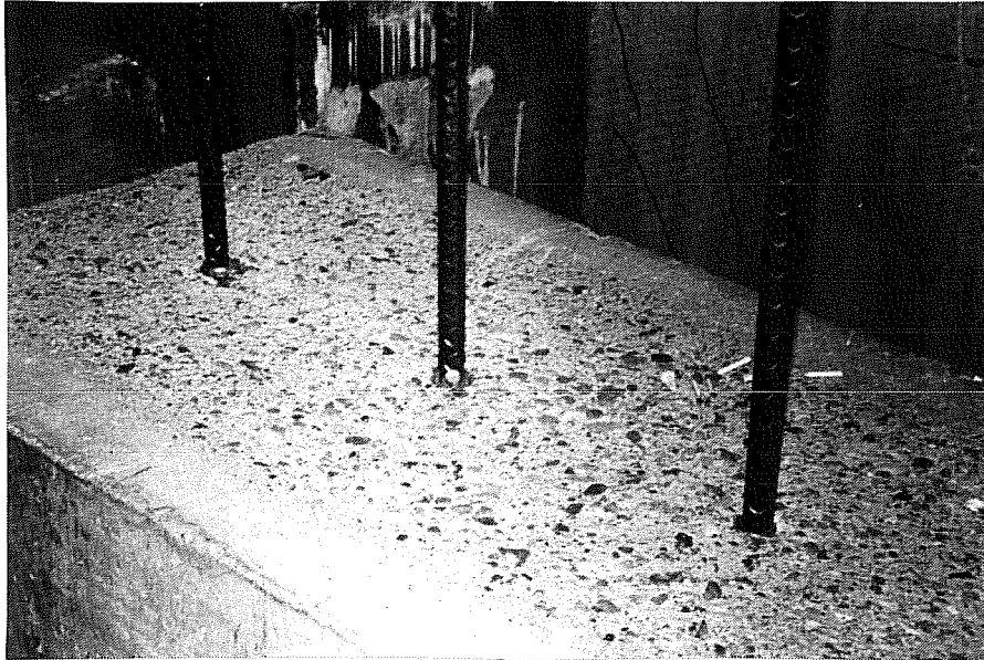
Fig. 3.25 Three #6 dowel bar arrangement for base block containing two #11 bars longitudinal reinforcement
