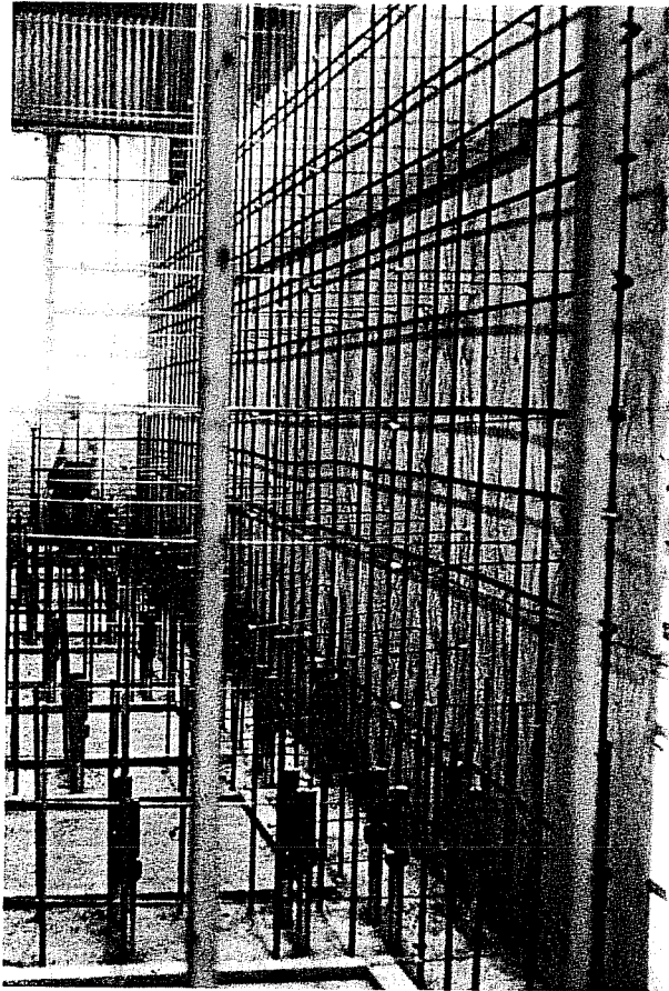
Fig. A14 Wall forms being erected with some wall steel in place
