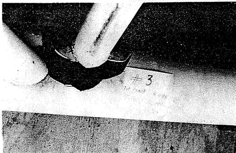
Fig. 4.3 Fatigue failure of K-3
