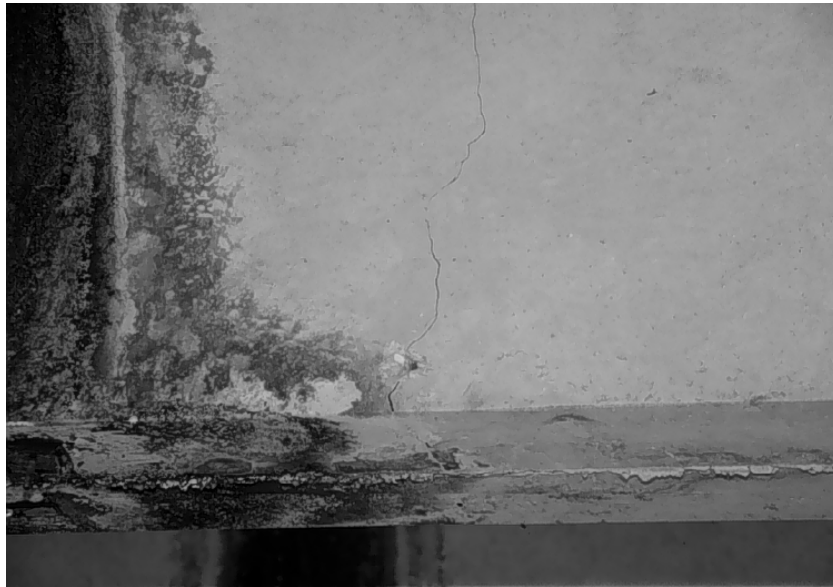
Figure 3.3 Vertical Crack in Girder
