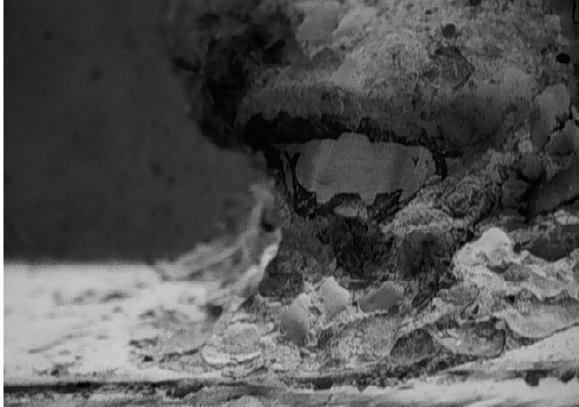
Figure 3.11 Exposed Reinforcing Bar at Midspan
