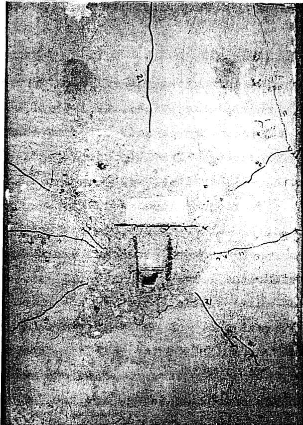
(b) Damaged cover removed
