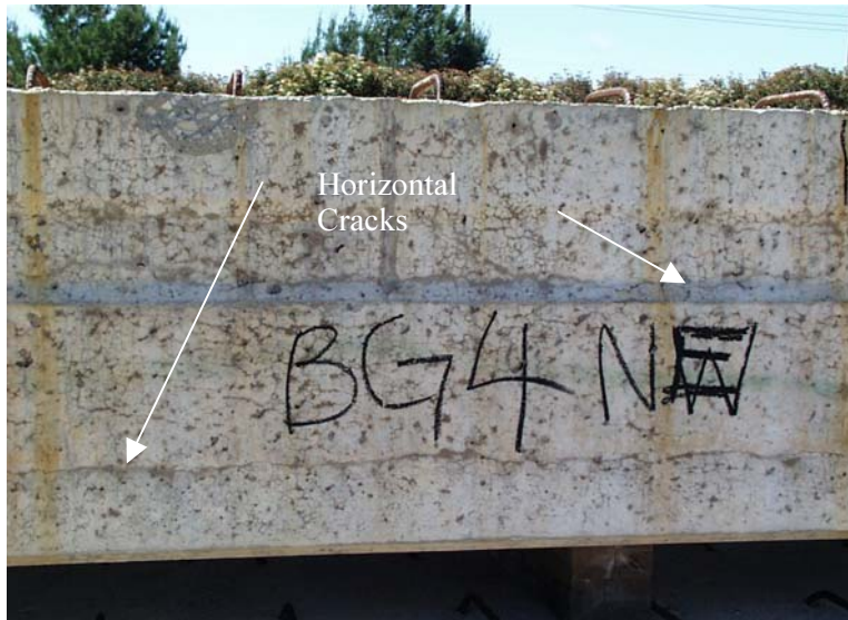
Figure 3.11 – Typical Damage along the Length of BG4
