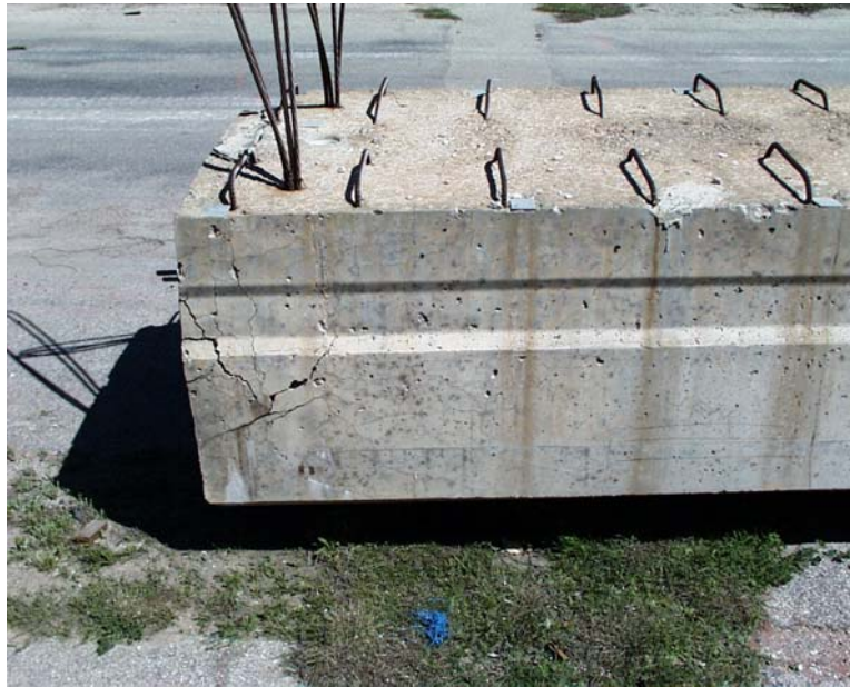
Figure 3.6 – End Damage on Specimen BG2
