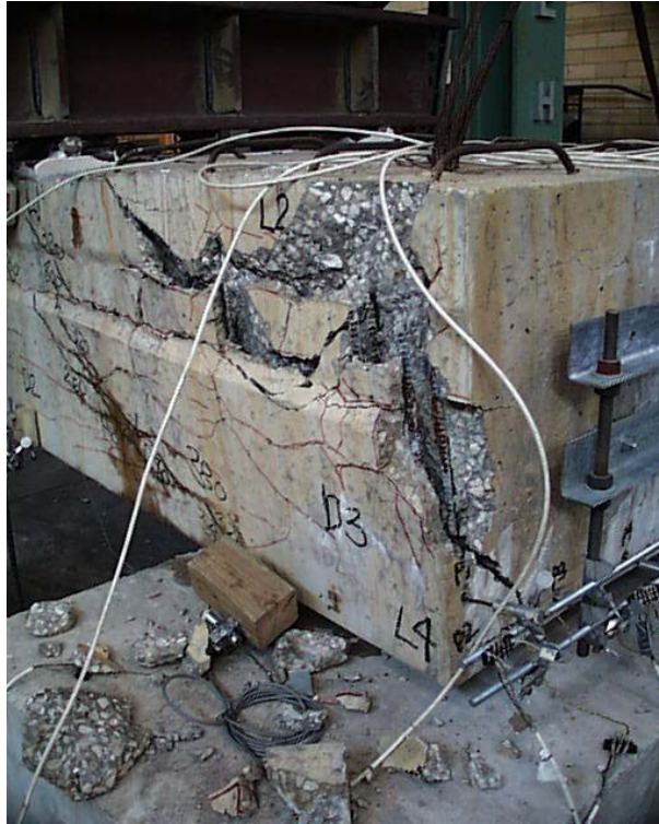
Figure 4.32 – Bearing Failure of BG4S
