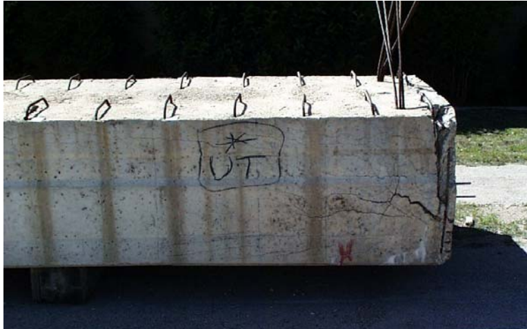
Figure 3.5 – Spalled Concrete on Specimen BG2
