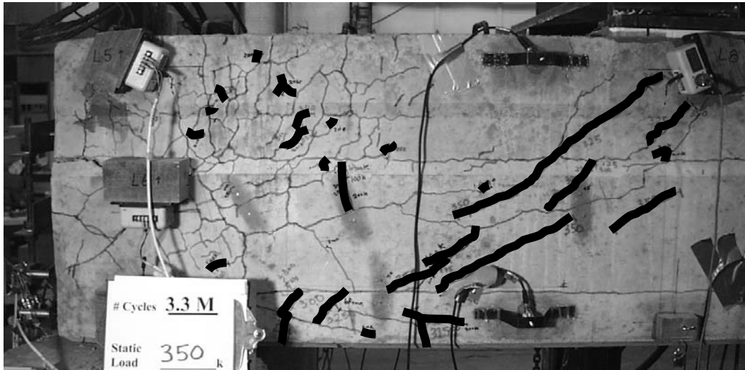
Figure 4.27 Shear-induced cracks in the east web of BG3S after 3,328,600 load cycles, and under a static load of 350 kips (1560 kN)
