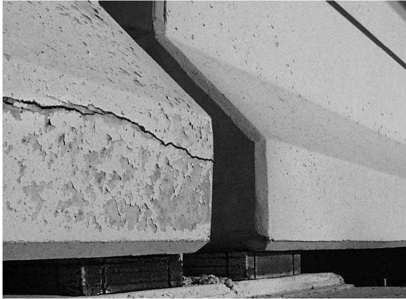
Figure 7.18 Contrast between damaged and undamaged girders at Location 1
