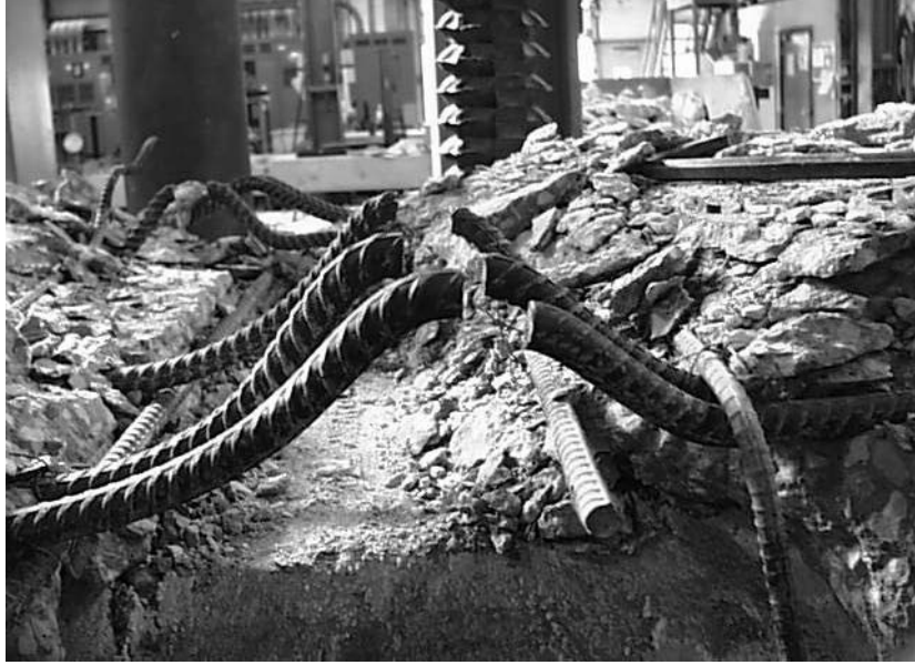
Figure 4.14 Fractured top reinforcement in BG4F
