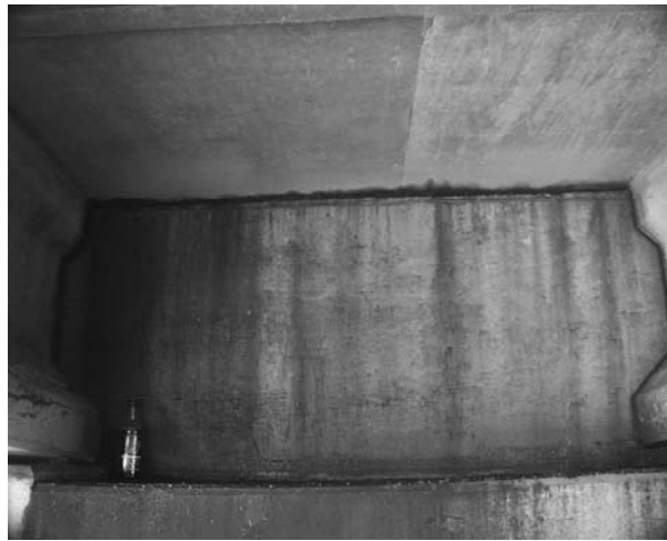
Figure 7.5 View of west abutment between SW Girder 2 (left) and SW Girder 3 (right)
