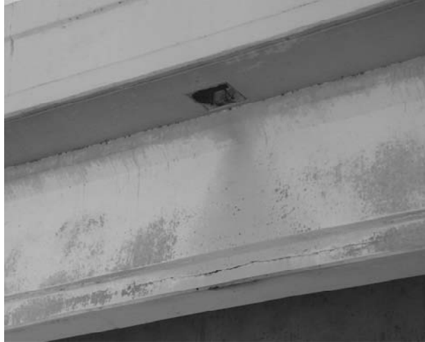
Figure 7.13 Cracking on Face 5 of exterior girder under drain scupper
