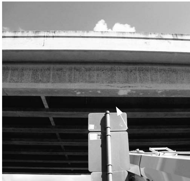
Figure 7.19 Cracks on Face 5 of exterior girder at Location 2
