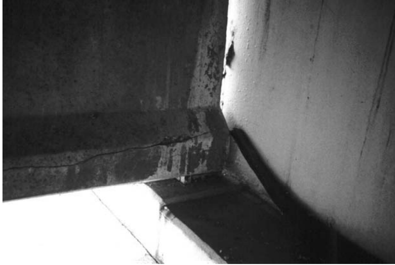
Figure 7.11 Rubber seal dropped from joint above at west abutment of US-90 structure
