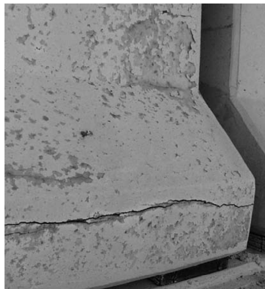
Figure 7.17 Typical cracks on bottom flange of Beltway 8 girders
