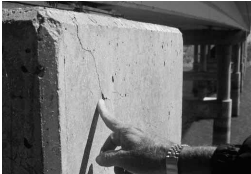
Figure 7.28 Map cracking at ends of bent cap (Bent 5)
