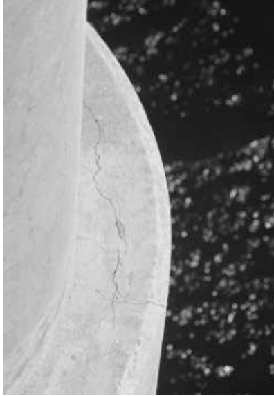
Figure 7.31 Propagation of vertical cracks in lower column to top of tie beam (Bent 5)
