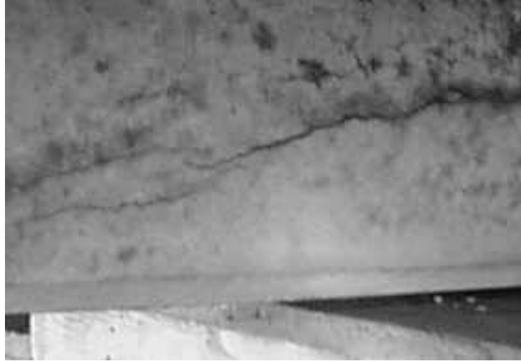
Figure 7.9 New cracks extending past the end of the old crack
