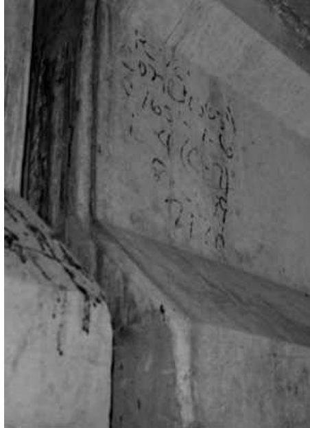
Figure 7.27 Horizontal cracking at bottom flanges of inside girder ends (Bent 5)
