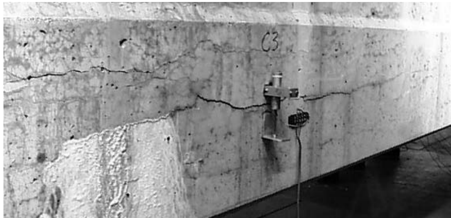
Figure 3.15 Linear potentiometer on west face of BG4F to monitor change in width of pre-existing crack
