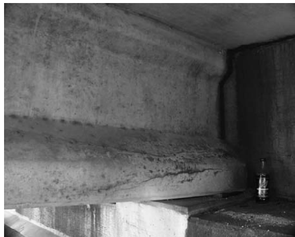
Figure 7.6 View of greater damage to SW Girder 2
