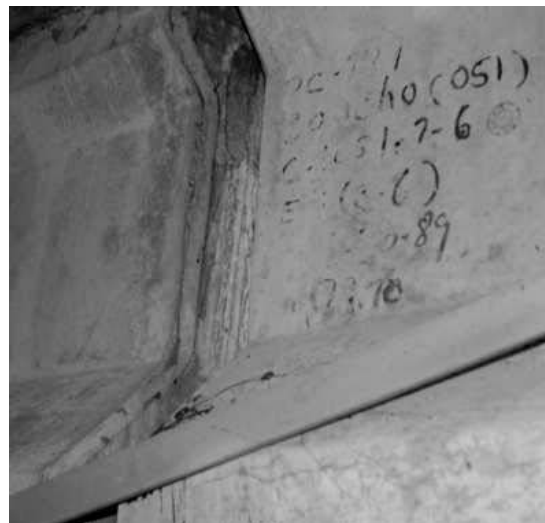
Figure 7.26 Horizontal cracking on bottom flanges of outside girder ends (Bent 5)
