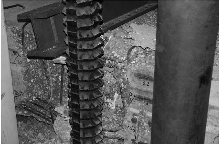
Figure 4.5 Flexural crack through Gages S3 and S4
