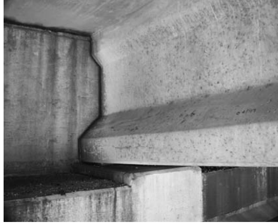
Figure 7.7 View of lesser damage to SW Girder 3
