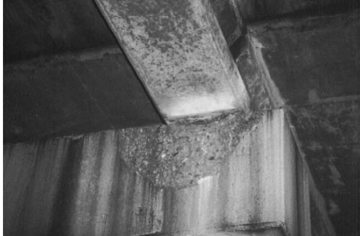
Figure 7.4 Missing bearing pad at I-10 structure
