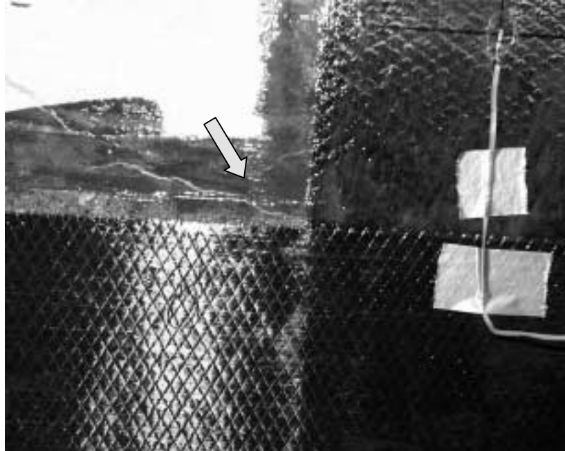
Figure 7.12 Initiation of Debonding Along CFRP Sheet
