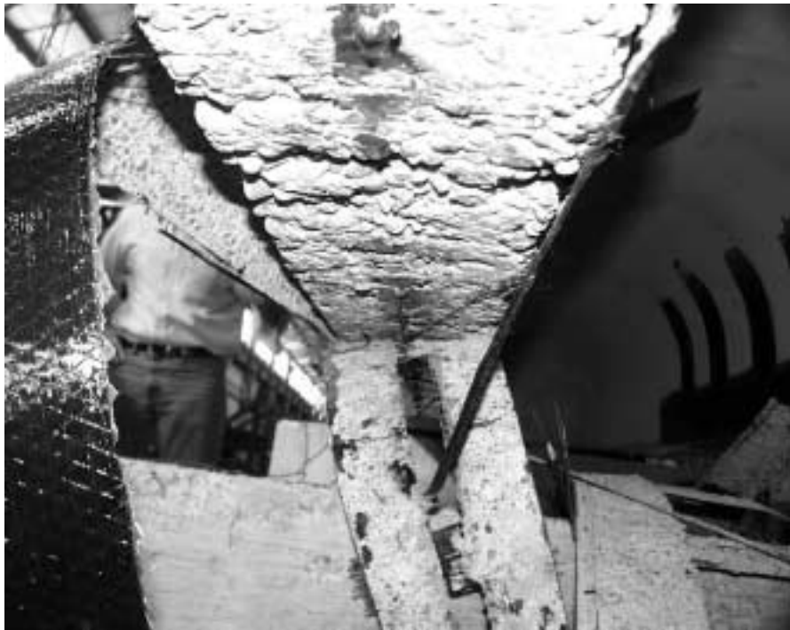
Figure 4.14 Bottom Surface Condition of West Joist after CFRP Debonding
