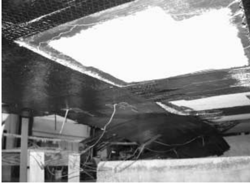
Figure 7.13 View of West CFRP Sheet after Debonding from Specimen FS-2
