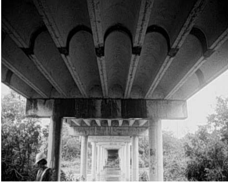
Figure 3.2 Photograph of Pan-Girder Bridge in Buda, Texas Indicating Uneven Surfaces on Bottom of Joists
