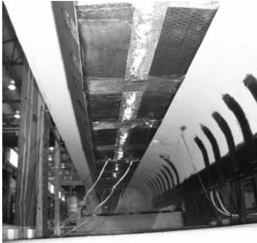
Figure 3.12 Partial Wrapping of Joists in Specimen J-2 to Avoid Concrete Surface Irregularities
