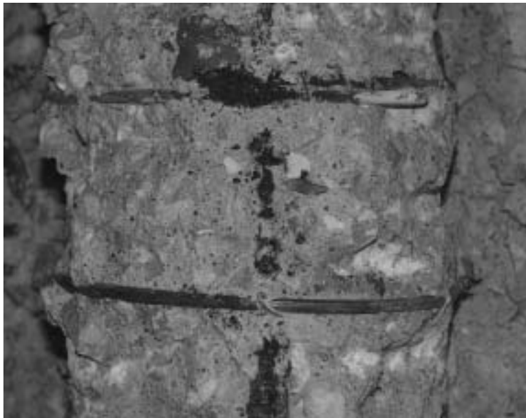
Figure 6.15 Macrocell formation in the top portion of specimen CC5
