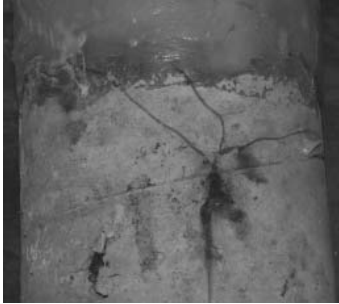
Figure 6.10 Evidence of corrosion activity in the splash zone of specimen CNC10
