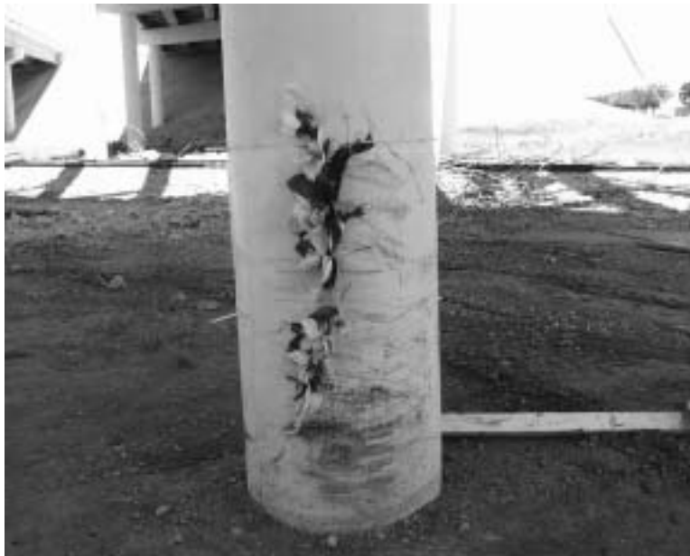
Figure 7.7 Vehicular collision damage on column of Structure #2
