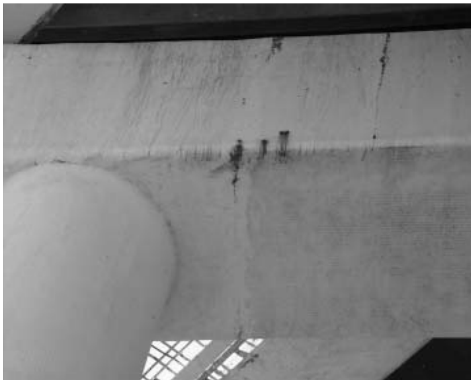
Figure 7.8 Rust stains on bent of Structure #1
