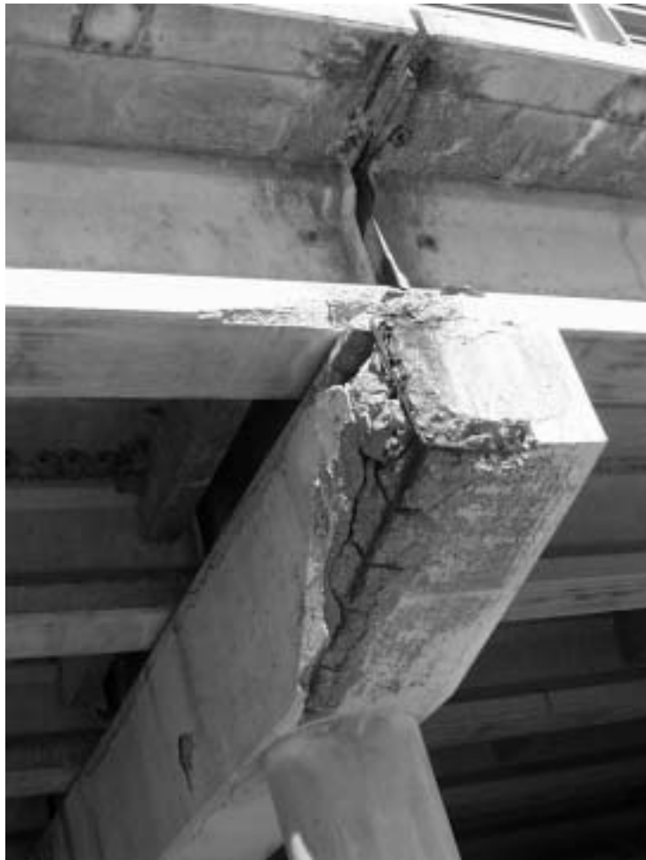
Figure 5.9 Delamination on an endcap of Structure #8
