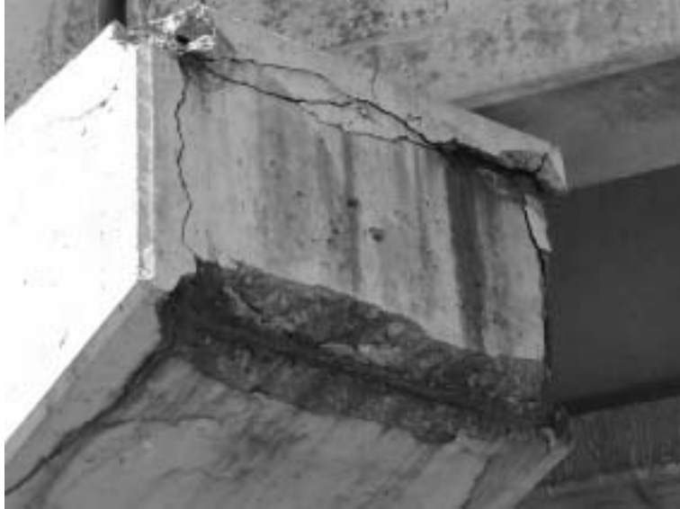
Figure 5.8 Damage to an endcap of Structure #5
