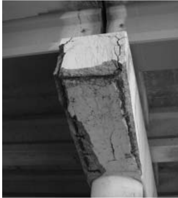
Figure 1.1 Corrosion damage to a bridge bent
