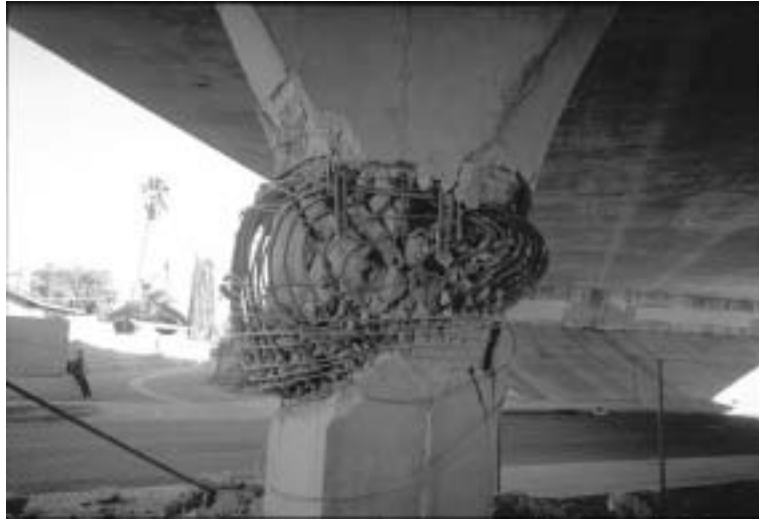
Figure 3.2 Highway bridge column after the 1994 Northridge earthquake (Courtesy of EERC, University of California, Berkeley).
