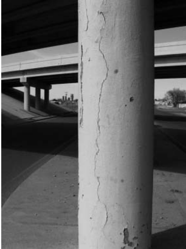
Figure 5.10 Cracking on column of Structure #12
