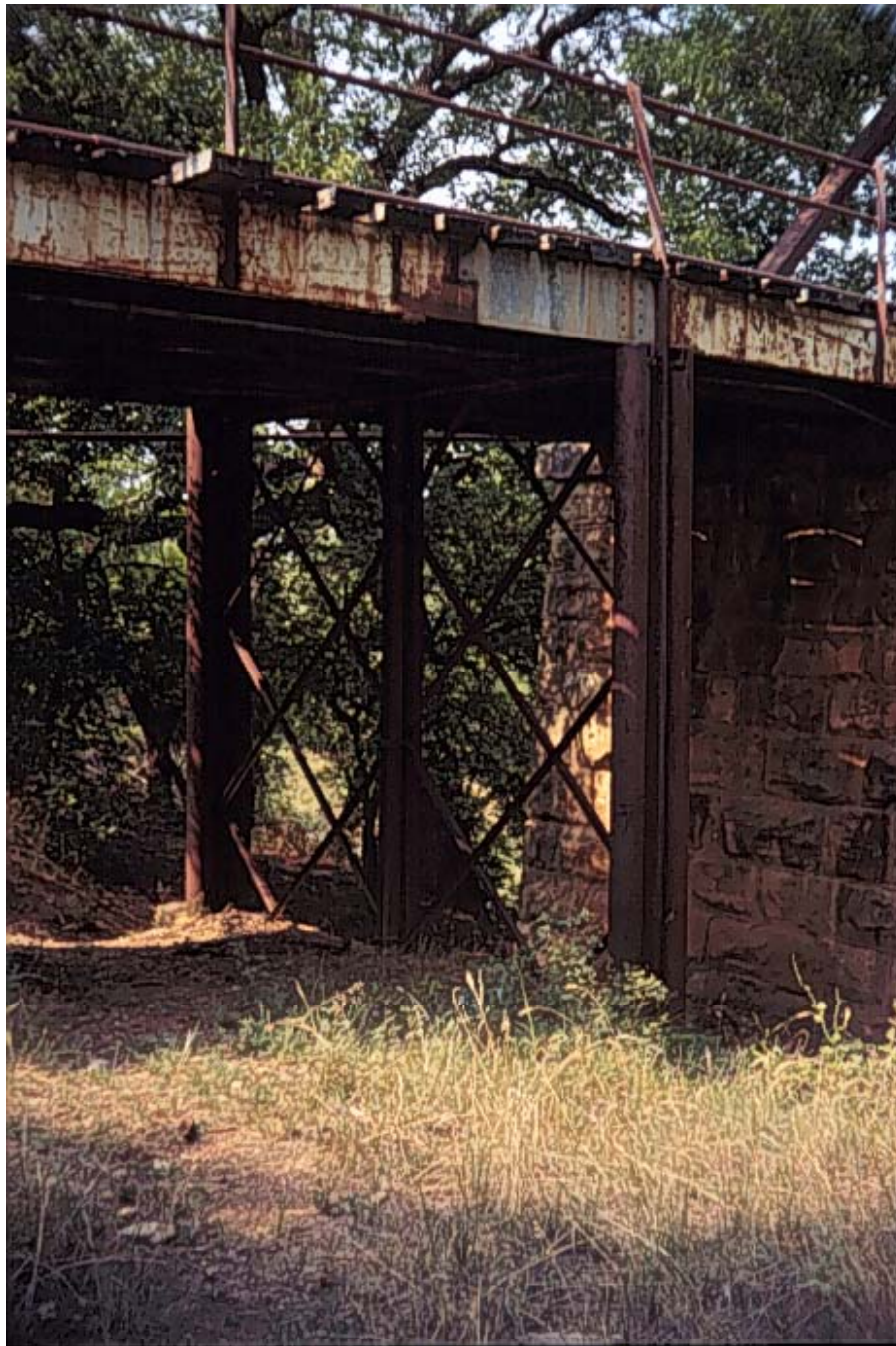
Figure A.26: Metal bent in the south approach span
