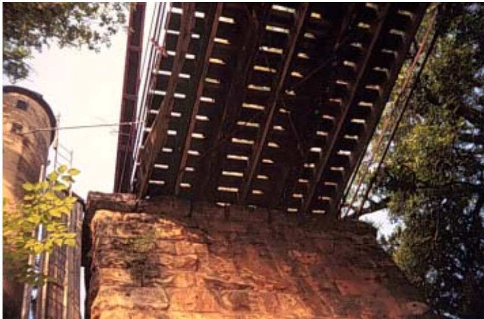
Figure A.29: Timber stringers of the main truss span resting on the south pier
