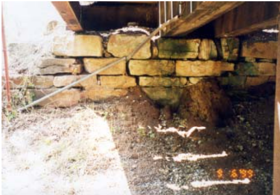
Figure A.35: Deteriorated abutment at south end of south approach span
