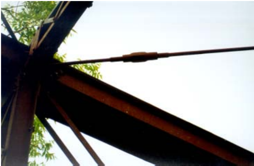
Figure A.22: Turnbuckle at a top bracing tension rod
