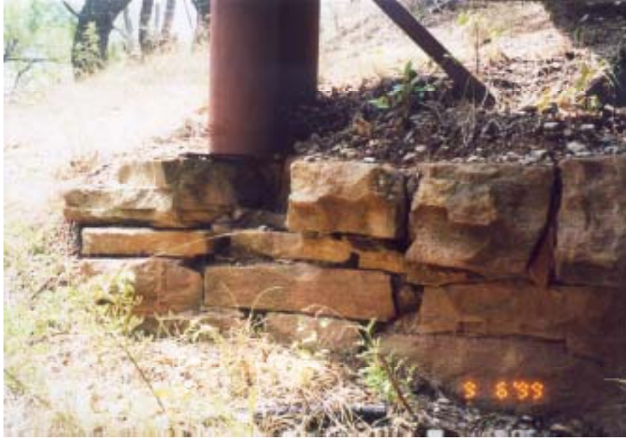
Figure A.32: Base of pipe column of metal bent for north approach span
