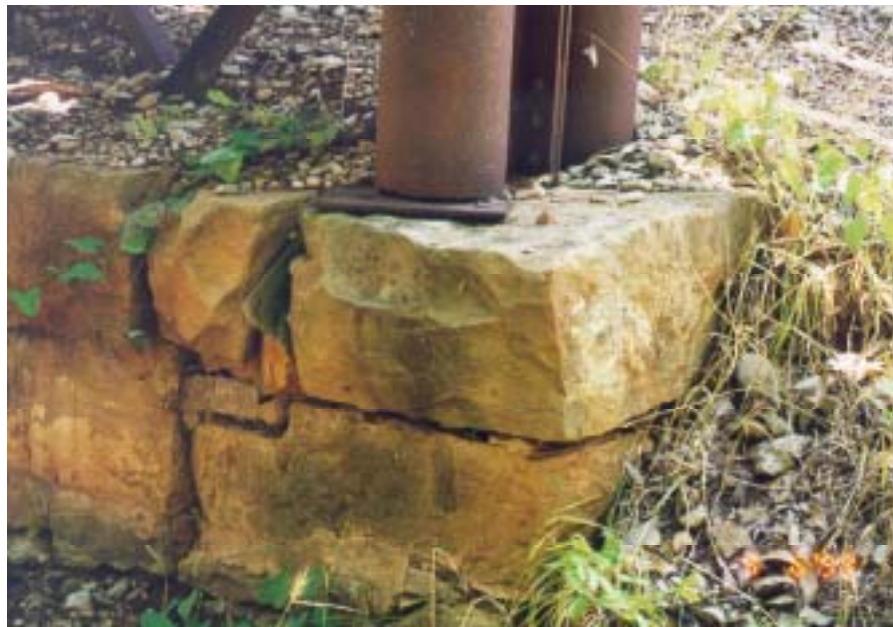
Figure A.33: Base of pipe column of metal bent for north approach span
