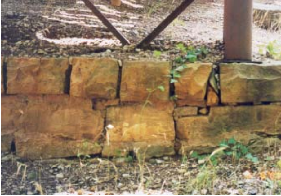
Figure A.34: Deteriorated foundation of metal bents for north approach span
