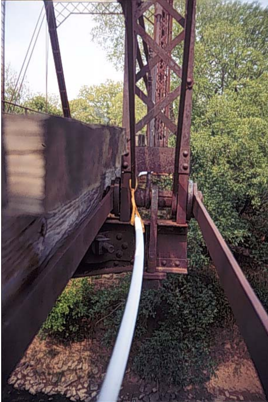
Figure A.10: Bottom chord joint L2
