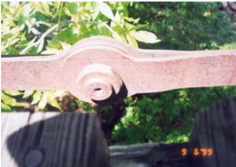
Figure A.12: Bottom chord joint L1
