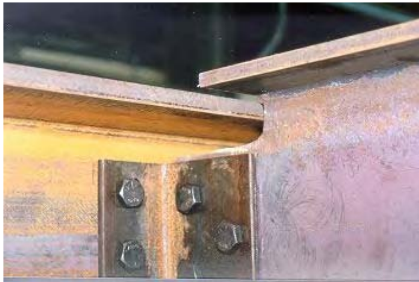
Figure 6.7 Cope detail showing elevated top flange of longitudinal stringer
