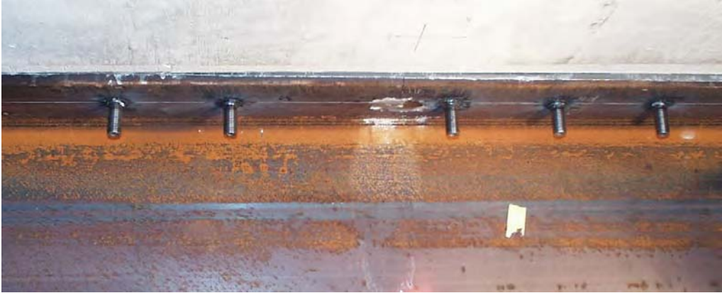
Figure 6.63 Threaded studs welded to the inside top flange of the transverse beam
