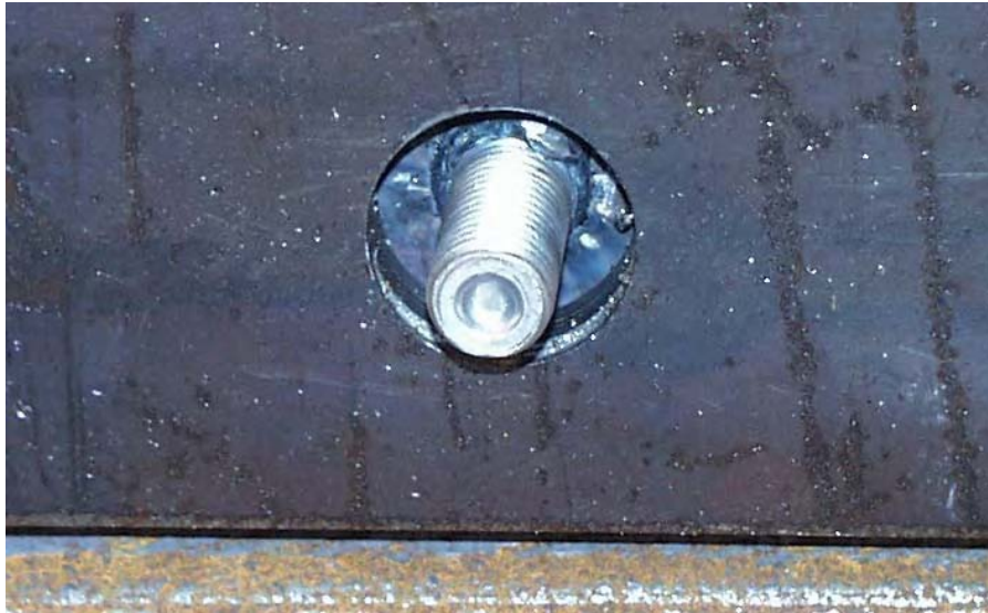
Figure 6.75 Gap around threaded stud
