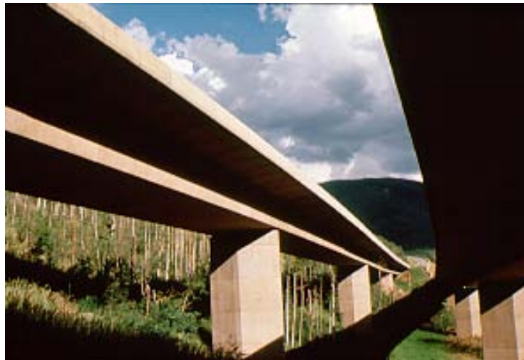
Figure 4.56 The concrete for these piers was stained to blend with the local rock coloring.
