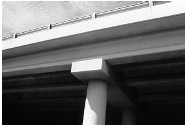
Figure 4.65 Inverted-T bent cap stem shaped to mimic the concrete I-girders it supports
