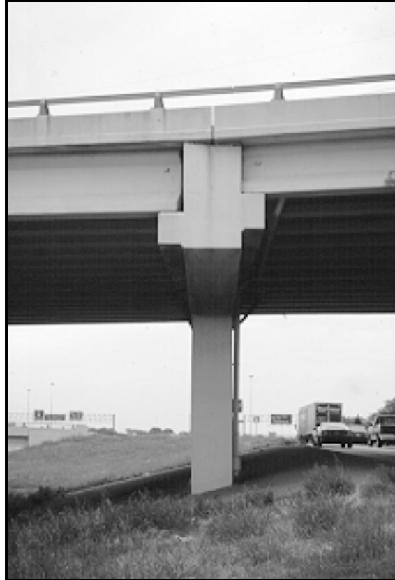
Figure 5.12 A change in superstructure depth highlighted by the awkwardly shaped bent cap end
