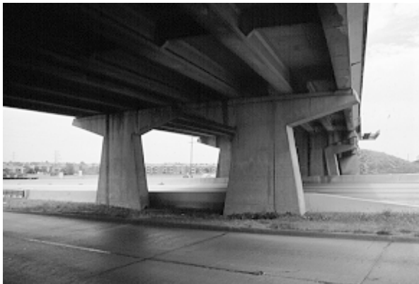
Extreme tapering in short substructure units exaggerates the flow of forces and appears contrived.
