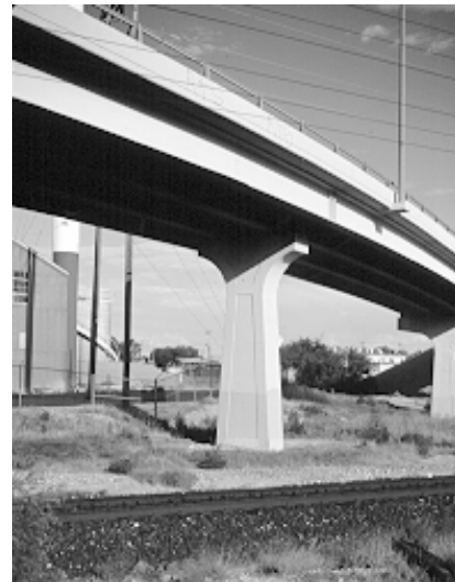
A flared column that stops short of the outer girders leaves the viewer with a sense of uneasiness about the support of the superstructure.
