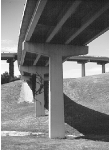
The tapered cap and column of this hammerhead bent is structurally expressive of the increased moment resistance required at the cap/column intersection and at the column base under critical loads
