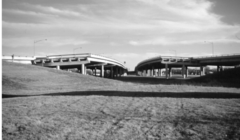
Figure 5.21 Stub-outs on the south end of the US 287 project (view looking south)
