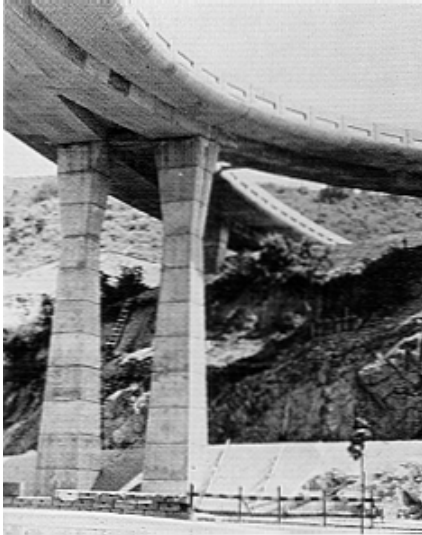
(a) These tall piers are more fixed at the base than at transverse the top. Under critical lateral loads, the point of inflection is located at about two-thirds the height from the base, allowing the columns to taper in at that location of minimum moment. [58]
