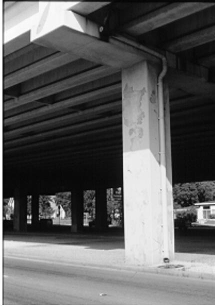
Figure 4.58 Unattractive peeling of painted concrete
