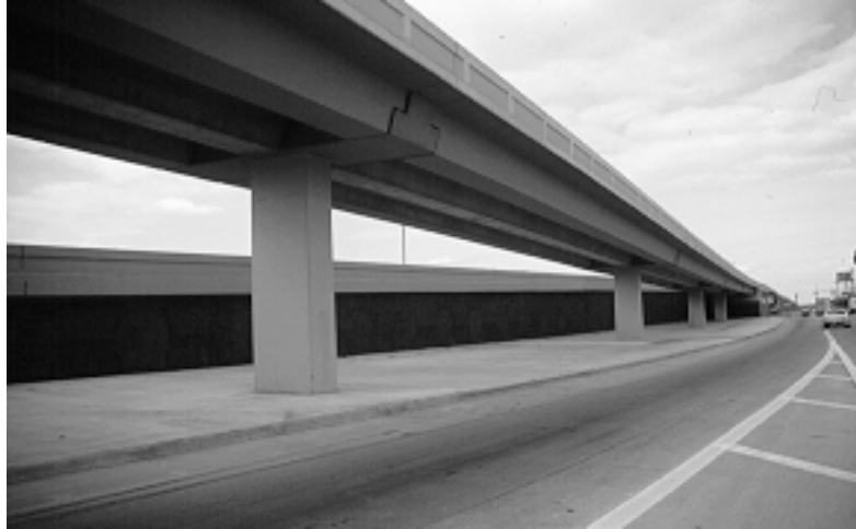
Figure 4.15 A hammerhead bent cap fully integrated into the depth of the superstructure through the use of dapped girders
