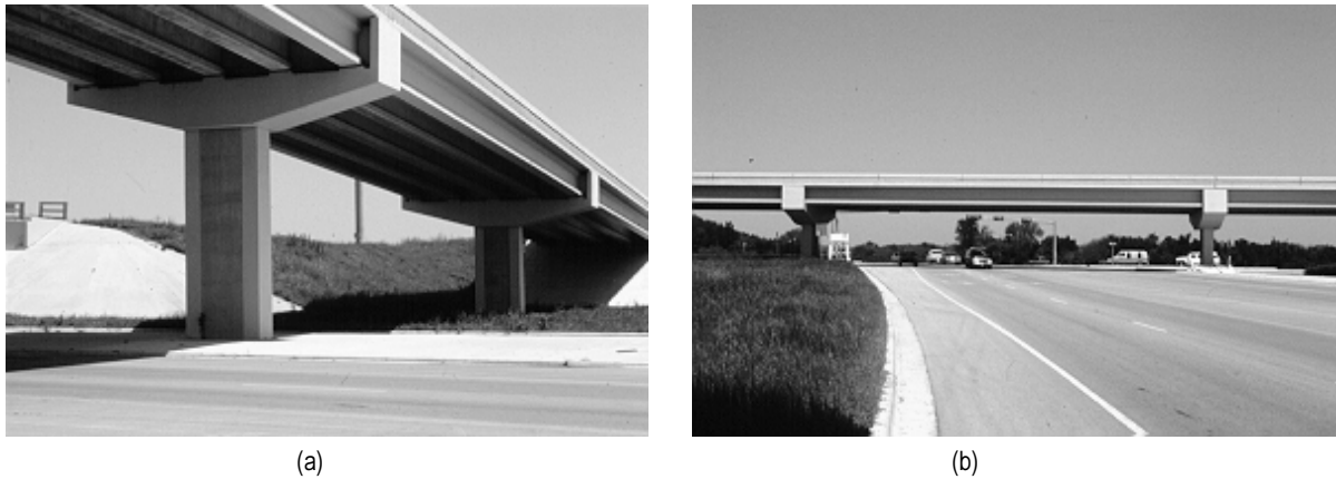
A thin wall at the end of a bent cap covers the gap between simply supported girders (a). The wall is unobtrusive in the oblique view (a) but gives the cap a disproportionately large appearance from the side (b).
