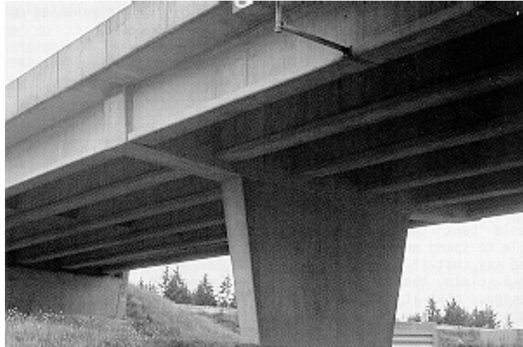
Figure 4.40 A fully integrated cap provides a clean transition between the superstructure and substructure
