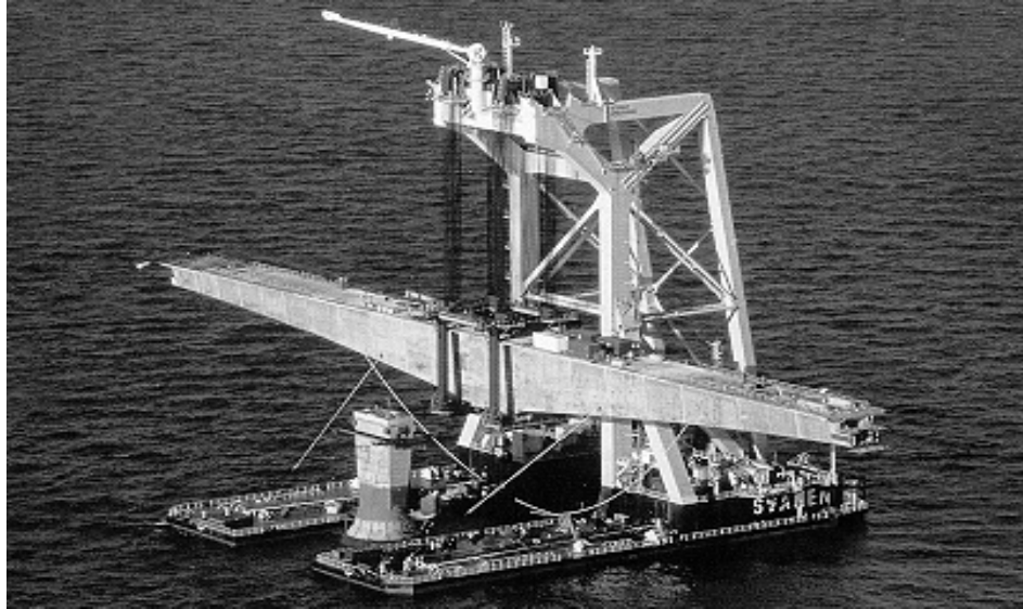
Figure 3.6 Placement of a 200 m (655 ft.) precast segmental girder for the Northumberland Strait crossing.[19] (Template segment is in position on top of the pier.)
