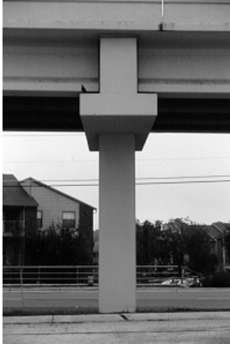
Figure 4.66 Balanced appearance of a column and bent cap stem of equal width
