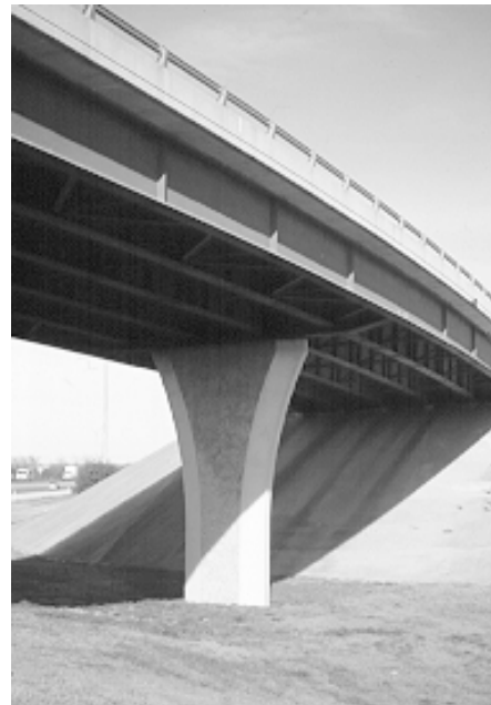
Figure 4.55 An elegantly tapered pier exposed aggregate used to accent slenderness; however, a disconcerting overall design—see Figure 4.23
