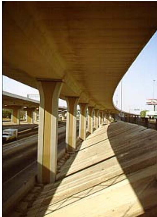
Figure 2.4 The San Antonio “Y” project in Texas shows off the elegance possible with segmental concrete bridge design
