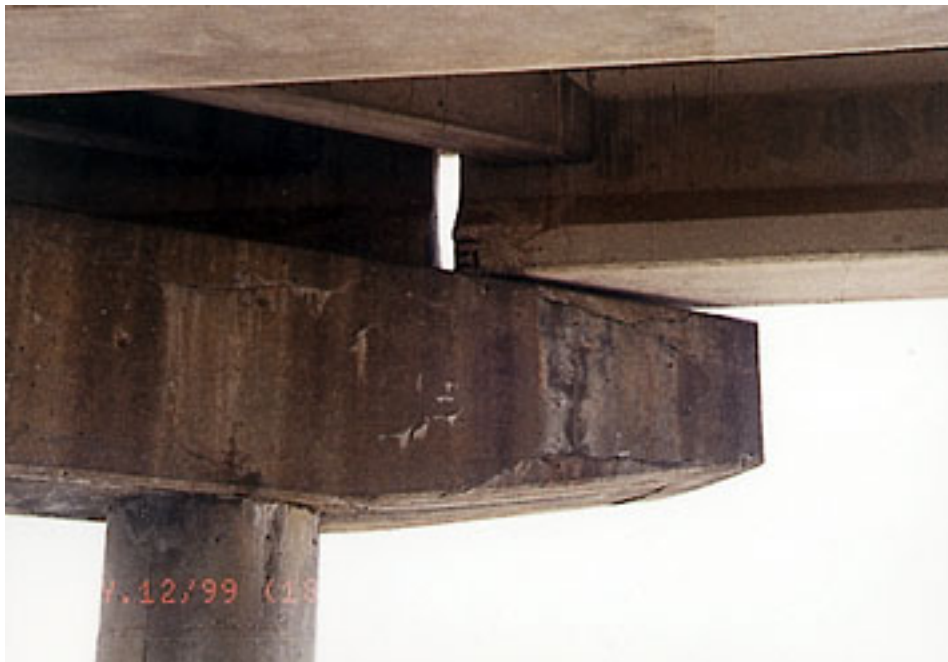
Figure 2.7 - Severe Deterioration of an Amarillo Bent Cap
