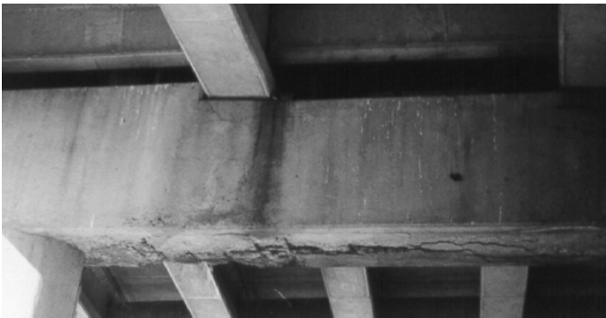
(c) Bent Cap Corrosion
