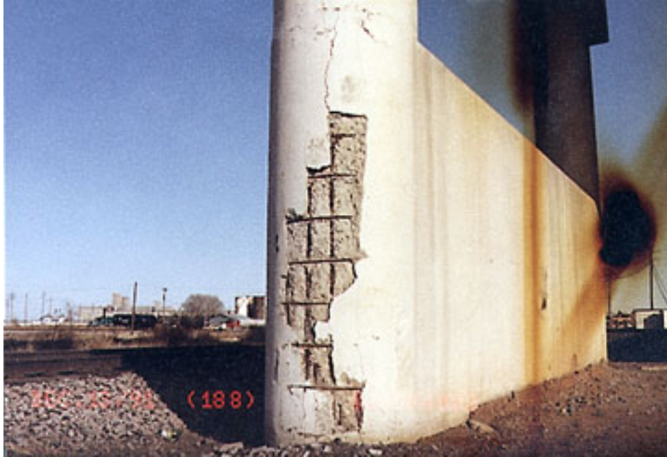
Figure 2.9 - Deterioration of Columns Due to Salt Laden Snow Piled against the Column
