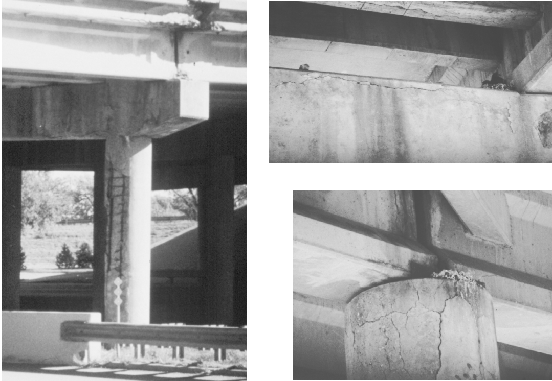
Figure 5.2 – Severe Substructure Corrosion Damage Due to Defective Expansion Joint
