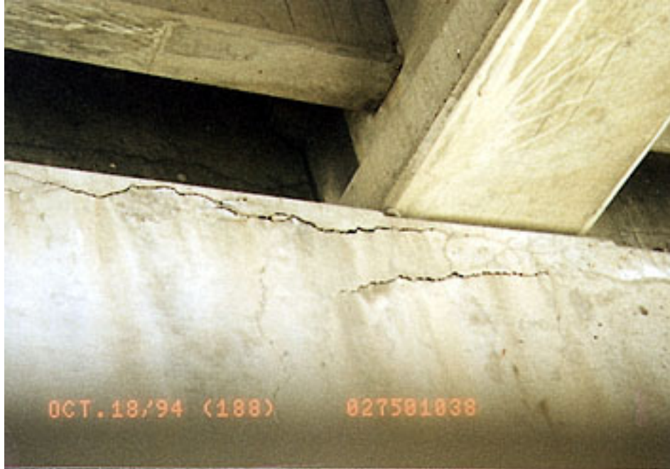
Figure 2.6 - Top and Side Splitting around Upper Reinforcement in Bent Cap (Amarillo)
