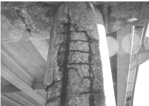
(b) Column Corrosion
