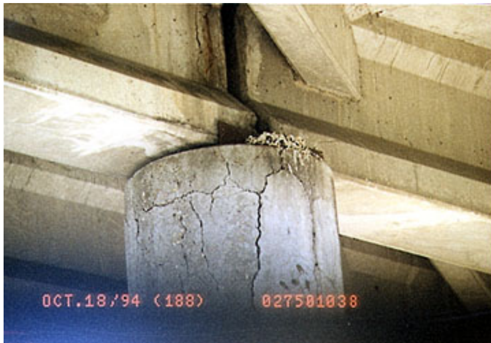
Figure 2.8 - Single Column Directly under a Construction Joint in Amarillo.
