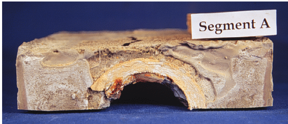
Figure 4.18 – Incomplete Epoxy Coverage in Epoxy/Gasket Joint (EG-S-M-NG-2)
