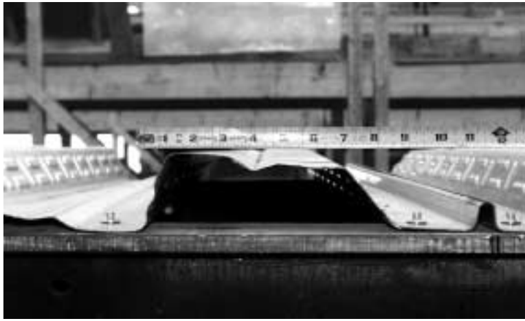
Figure 8.2 Metal Deck Distortion
