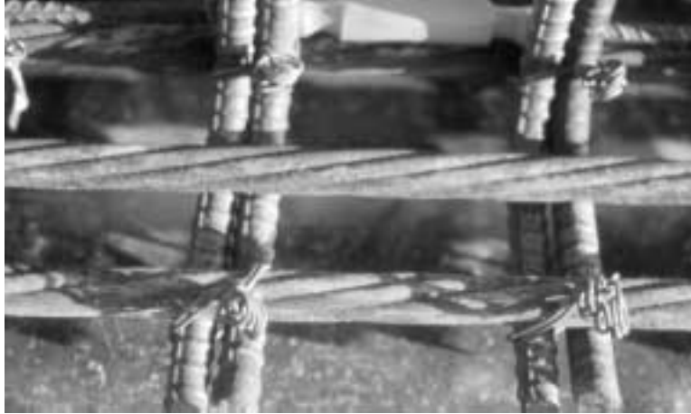
Figure 3.11: "Rusted" Strand Surface Condition
