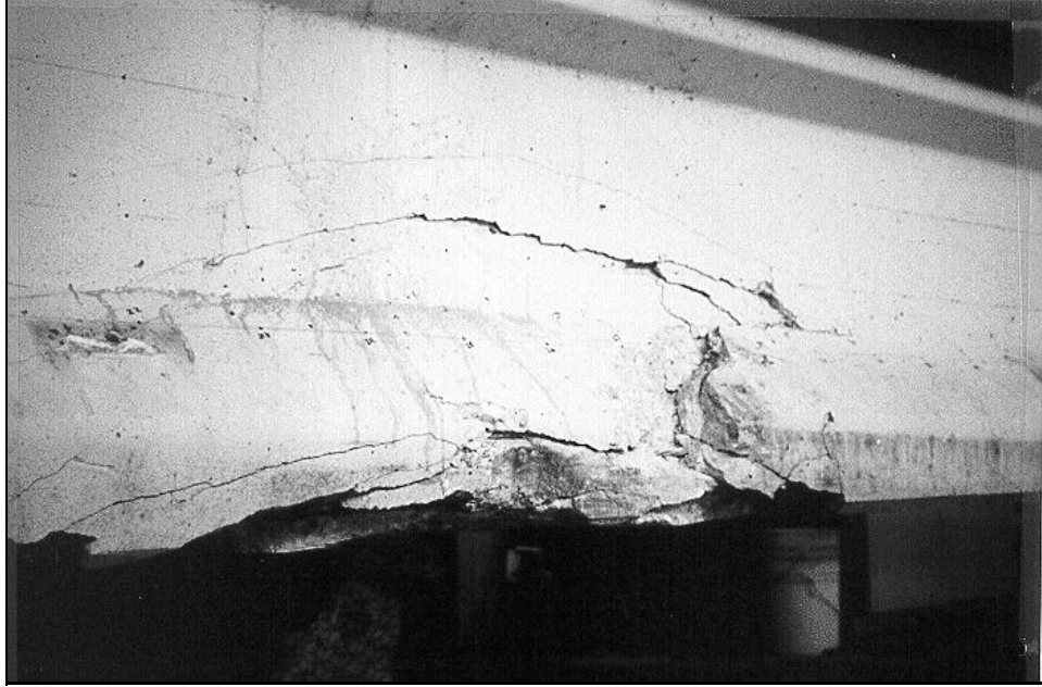
Figure 7- 8 Example of side impact damage to concrete
