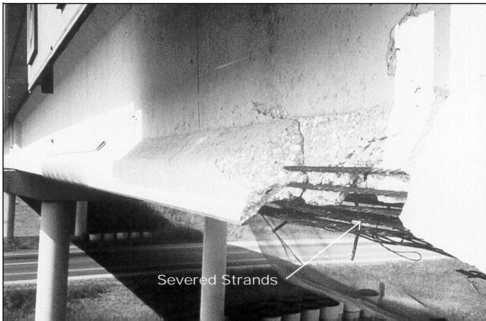
Figure 7- 9 Large volume loss of concrete cross section
