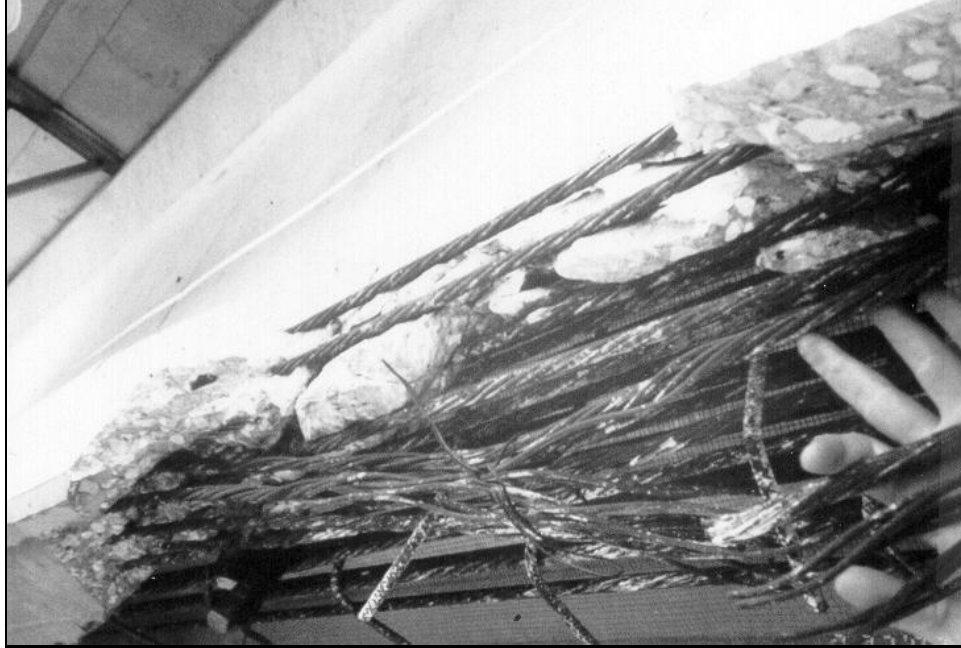
Figure 7- 14 Misalignment and complete severing of strands
